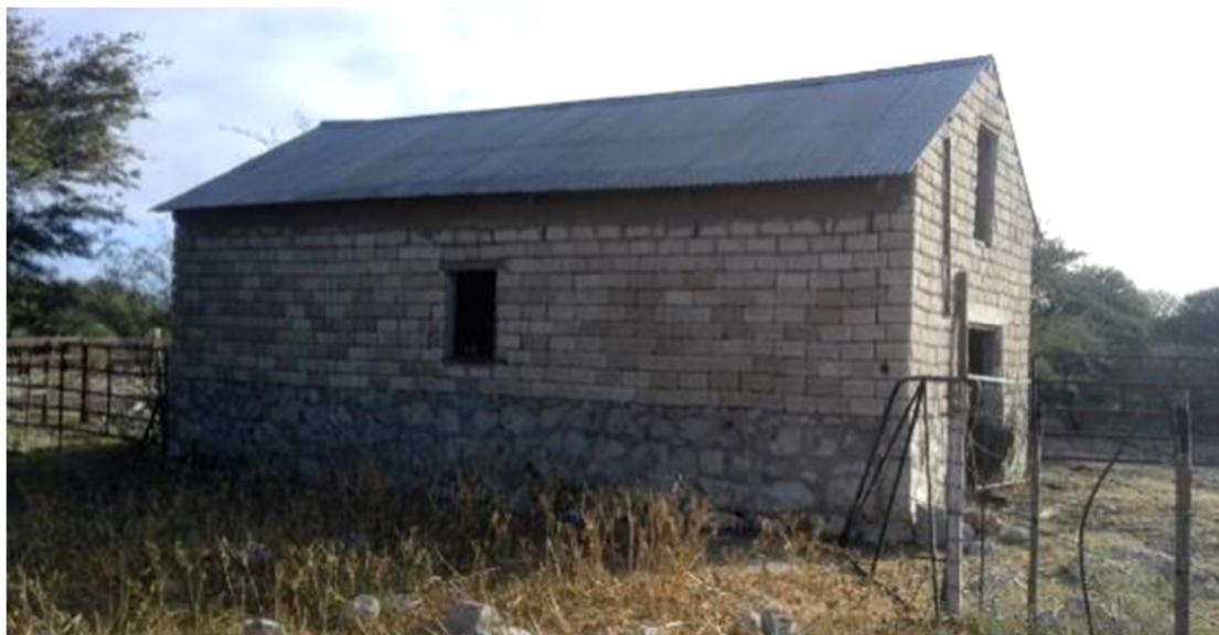
Fig. 40. Apart from the graves on Bergville this milking shed is most probably the most important heritage relic on the farm. It is difficult to actually date it on architectural features only. It is certainly related to the construction of the reservoir and the early part of flood irrigation. Very few of this type of structures survive in the general area. This is a protected building under the heritage Act. (North elevation.) (Photo S.M. Miller 2018.)
