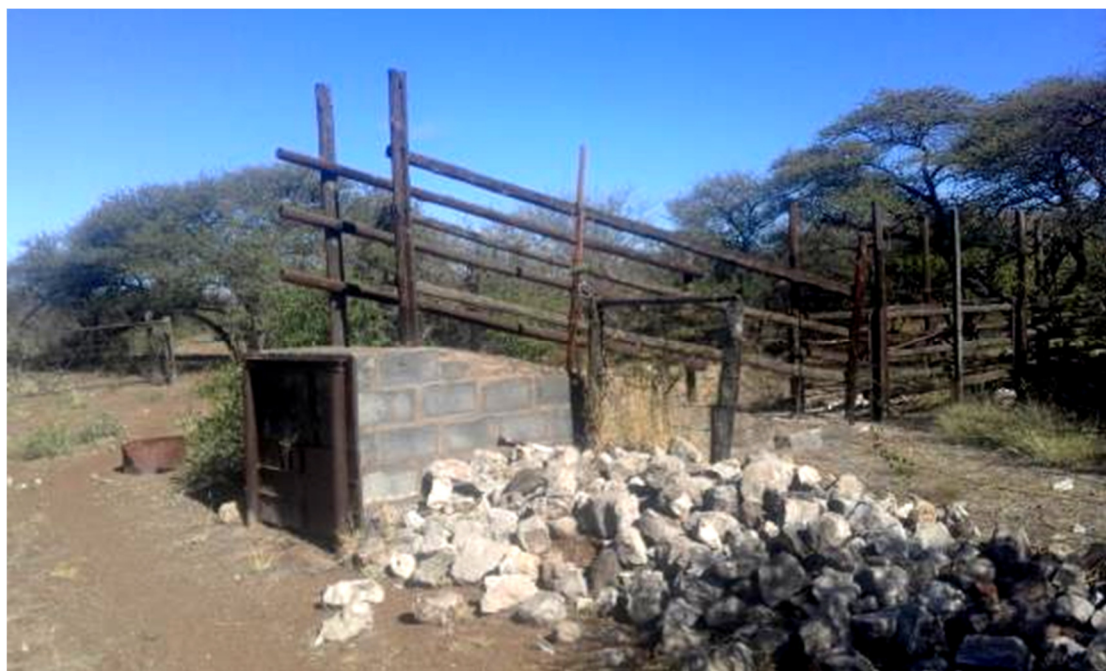
Fig. 64. Cattle loading platform adjacent to the Ghaap station. This is a modern construction but the limestone blocks suggest that there was an earlier structure year as well. (Photos S.M. Miller 2018.)
