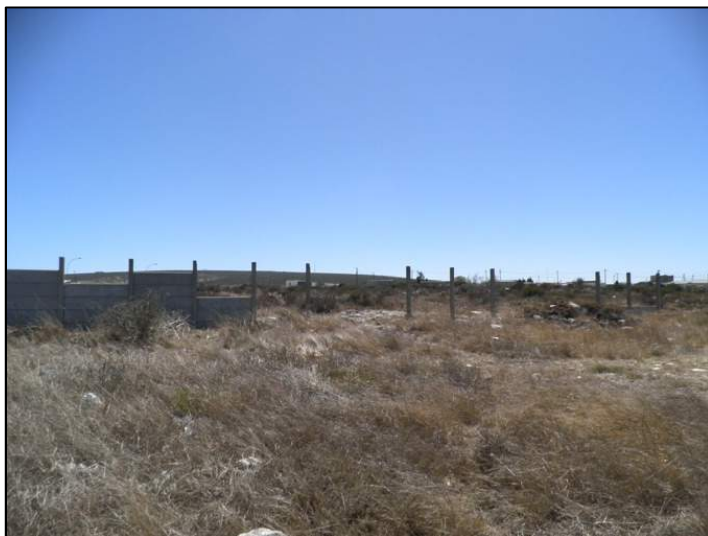
Photograph 3: Existing vibracrete wall that has been vandalised and stolen.
