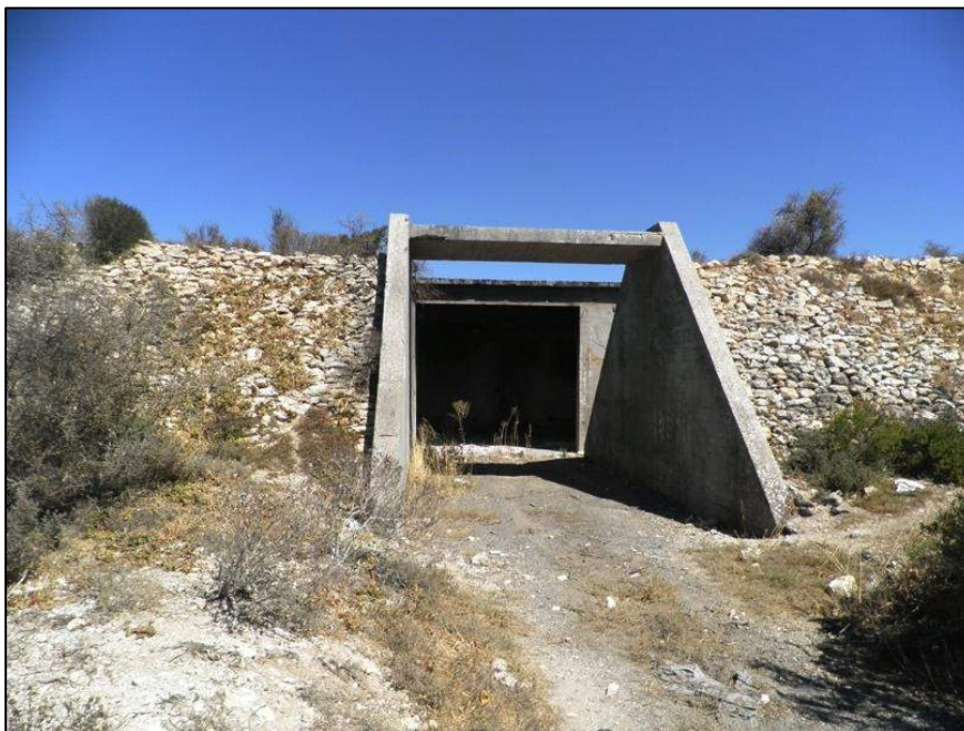
Photograph 3.1: Saldanha Military site: one of two bunkers dating from WW2. The steel door to the entrance of the bunker has been stolen. The bunker is sued for vandalised (refer photo below) 2013 O'Donoghue
