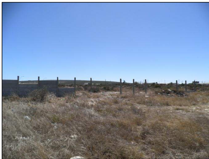
Photograph 2.10: Saldanha Military site: existing vibracrete wall that is vandalised and stolen defining site and municipal land; position of proposed wall, 2013 O'Donoghue
