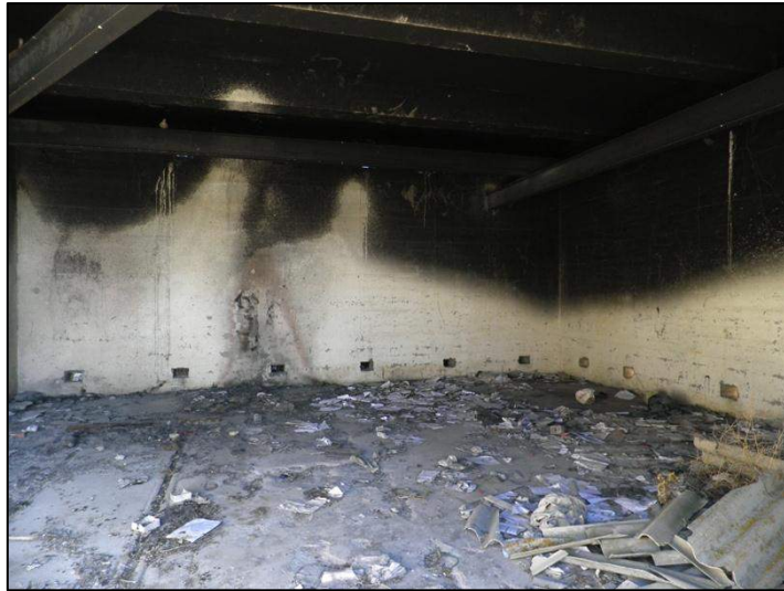
Photograph 3.2: Saldanha Military site: interior of one of two bunkers dating from WW2. The steel door to the entrance of the bunker has been stolen. The bunker is sued for vandalised (refer photo below) 2013 O'Donoghue
