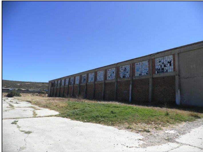
Photograph 2.15: Existing structure (hall) constantly damaged by local residents. Mrs Mkebi reportedly hosted a major event at this venue c 2007 when the building was in excellent condition, 2013 O'Donoghue
