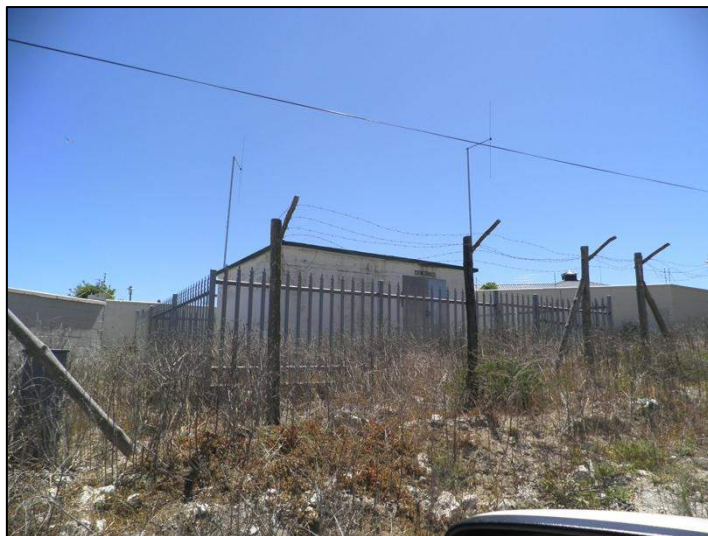
Photograph 2.23: Example of steel palisade fence erected around municipal substation to prevent theft and vandalism. Reportedly this palisade fencing is not considered to provide sufficient security, 2013 O'Donoghue
