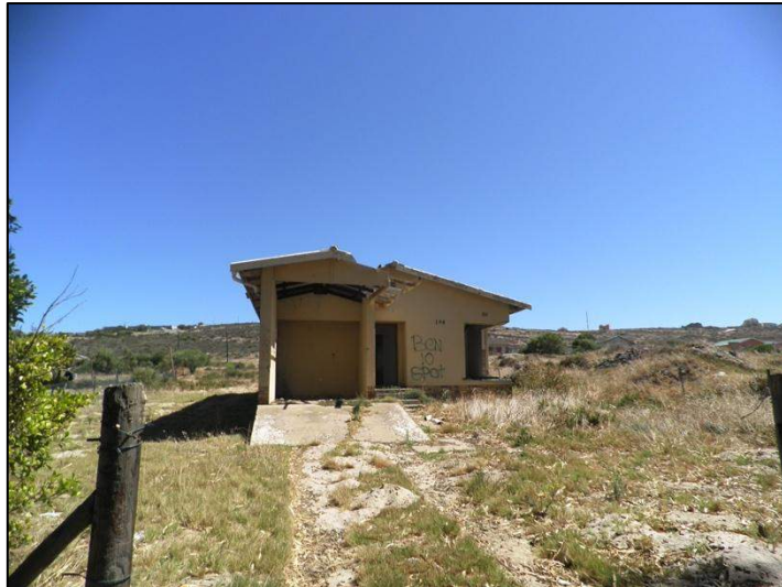
Photograph 2.18: Saldanha Military site: Existing structure (residence) that has become inhabitable due to theft and vandalism, 2013 O'Donoghue
