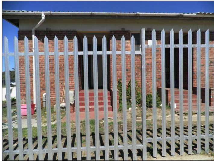
Photograph 2.24: Example of steel palisade fence erected around the clinic to give protection to staff, their vehicles and the building, 2013 O'Donoghue
