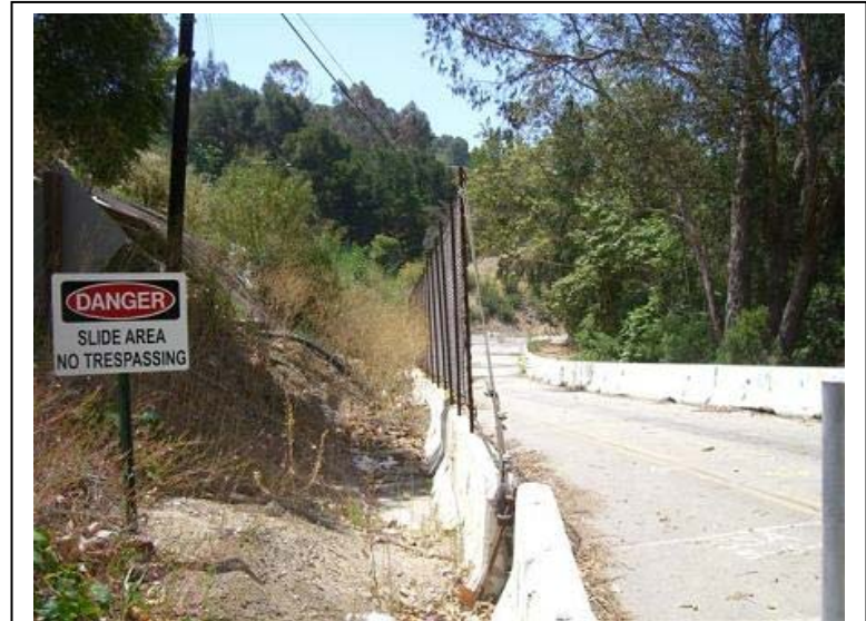
The Sycamore Canyon landslide has led to the semi-permanent closure of State Highway 144 (Photo from the Santa Barbara Independent 2007).
