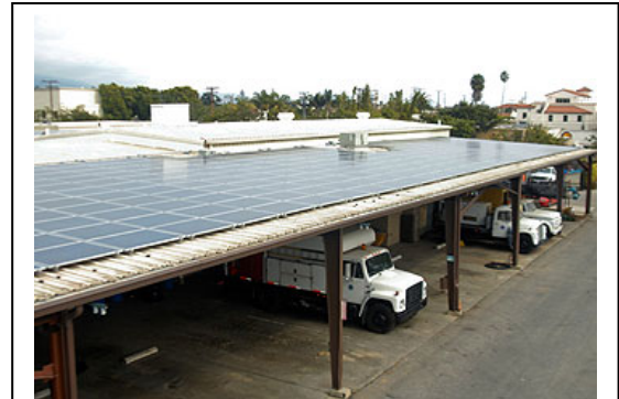
The city of Santa Barbara recently installed a 384 kw solar facility that supplies some City buildings with renewable power.
