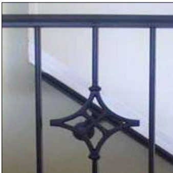
WROUGHT IRON RAILING/GRILLE BENJAMIN MOORE Black Panther 2125-10 COLOR SUBJECT TO FIELD VERIFICATION
