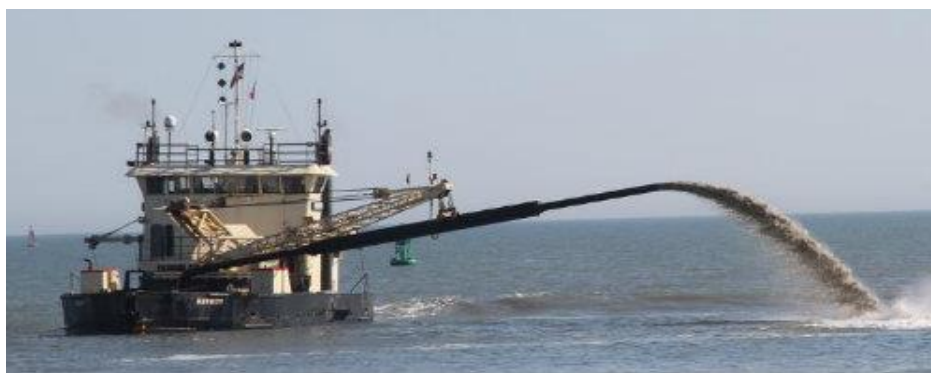
Photo 3.3. View of sidecast dredge, the Merritt, working within the outer bar channel of LFI.
