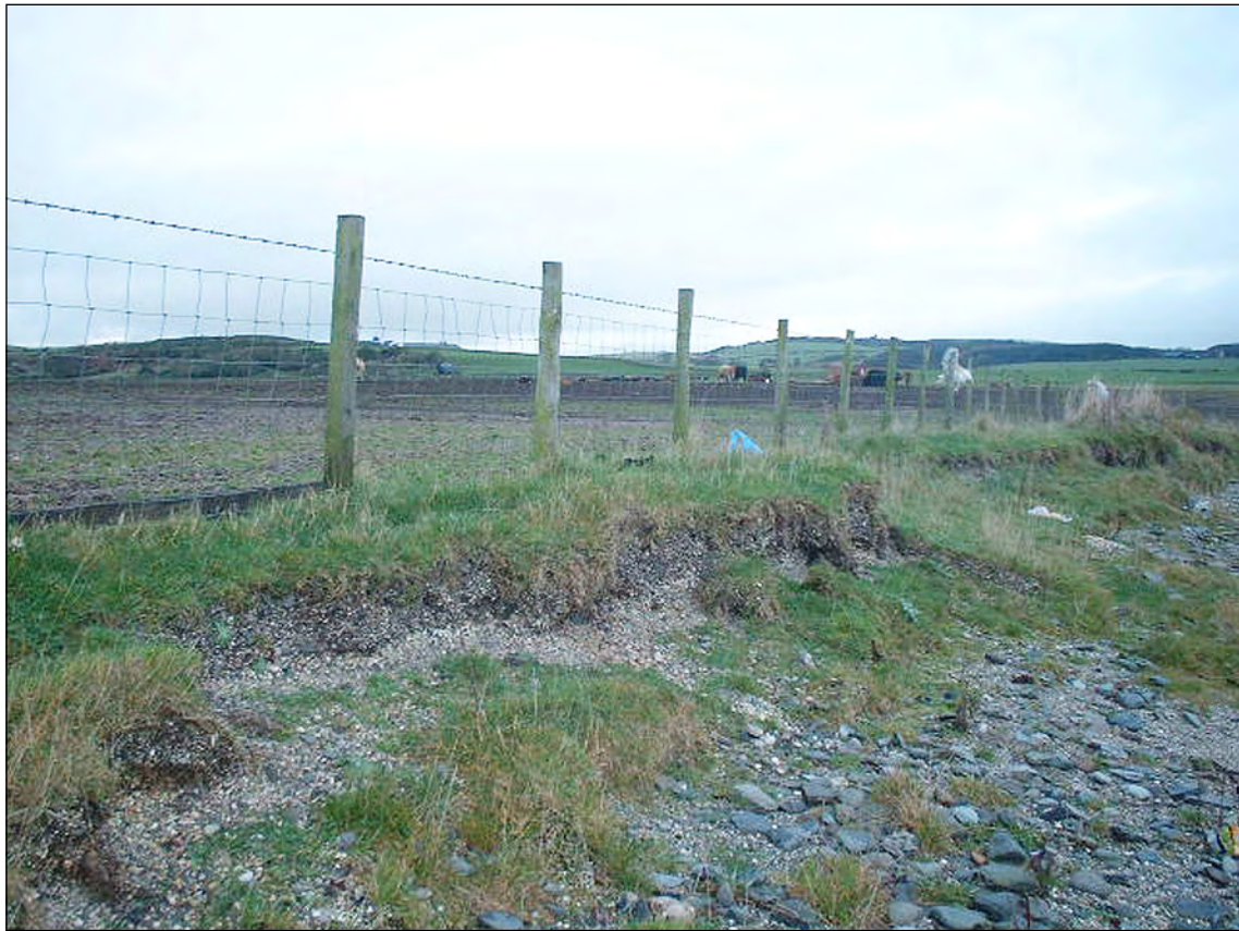
Plate 5 - Eroding marine deposits at St Ninian's Bay on the west coast of Bute. (Unit 2, Erosion Class, Bute Map 8)
