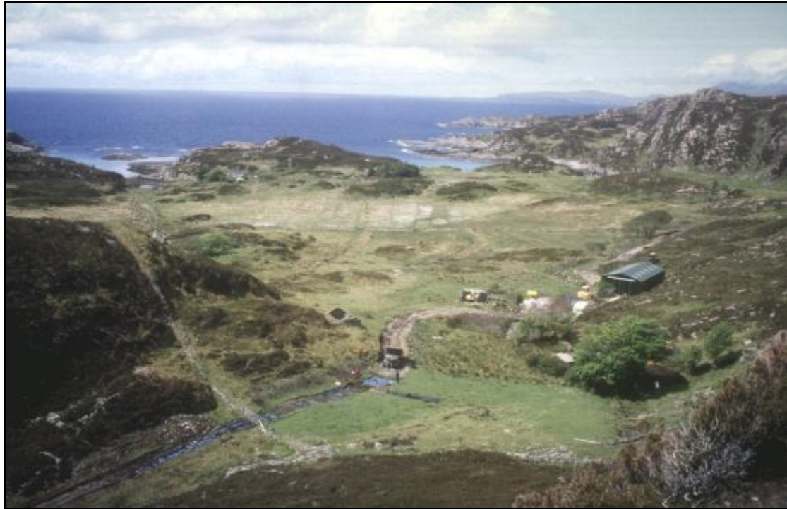
Figure 9: The excavation site at Camas Daraich, Skye. Note site trench in centre foreground, in front of lorry ©Caroline Wickham-Jones
