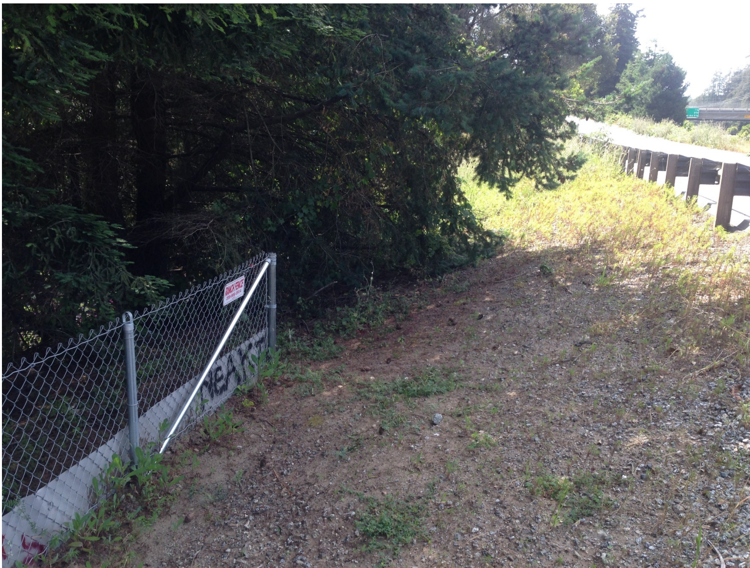
Figure 5. Photo showing the northern end of the exclusion fence near Rio Del Mar Boulevard. Note the open access to the shoulder.
