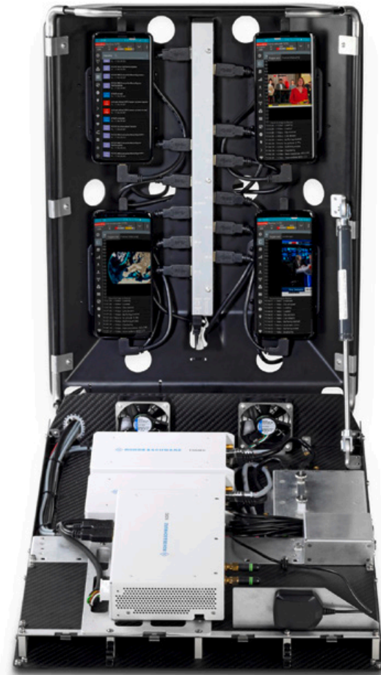
View of inside with QualiPoc, R&S®NCM2 compact integrated PC and R&S®TSMx6 ultracompact drive test scanner
