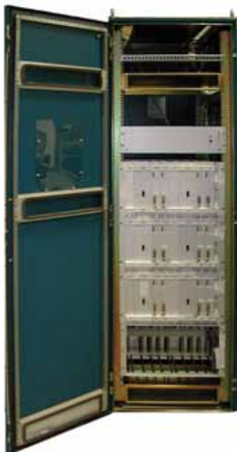
Application: Control system
