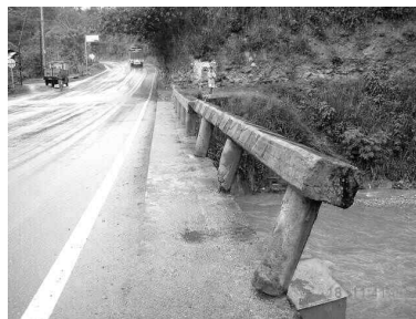
Figura 9. Barandas inestables por impacto Figure 9. Unstable safety fences due to collisions
