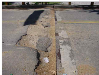
Figura 6. Falla unión soldada en junta de acero. Soldaduras intermitentes Figure 6. Welding failure of steel joint. Non continuous welding
