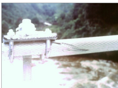
Figura 40. Catenaria principal con falla en alambres Figure 40. Main catenary showing wires failure
