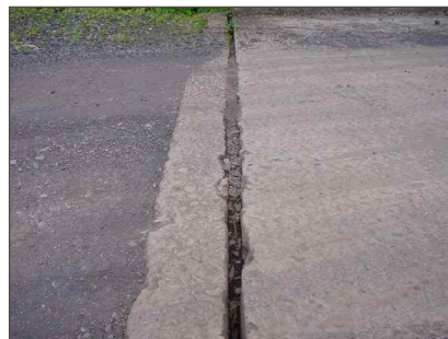
Figura 4. Junta sin sello y cubierto con tierra Figure 4. Joint lacking of pier ring, covered with earth
