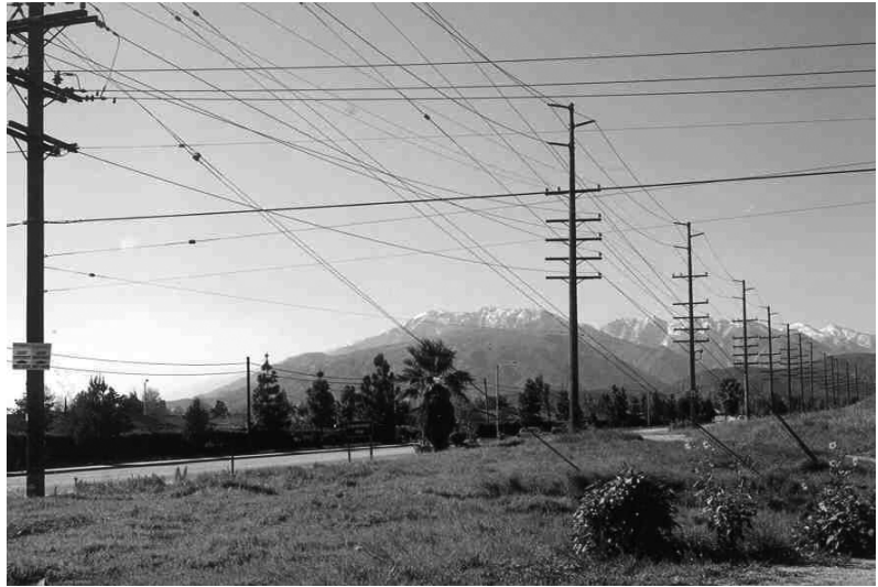
Accommodating urban infrastructure to support growing populations is a management challenge (Cleveland NF photo).
