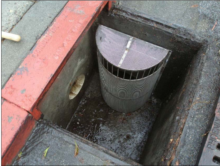
Figure 2.2. Example small full-capture device used as a monitoring site.
