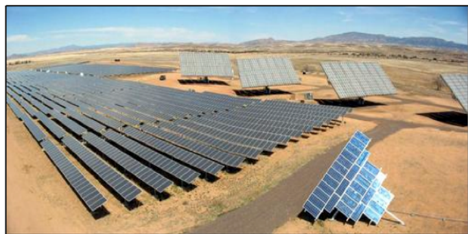
Figure 5.1 Existing Amonix CPV System in Arizona. Source: Arizona Public Service Commission.
