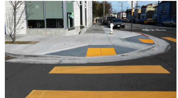
Accessible crossings meet code
