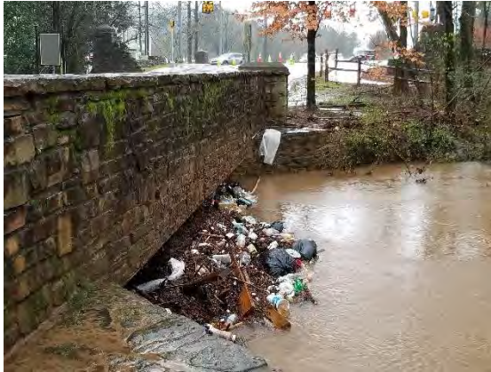
Figure 5.3: Trash under bridge in Shades Creek
