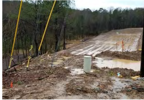
Figure 5.1: Erosion and Sediment Runoff Post Rain Event on Bulldozed site, Shades Creek Watershed
