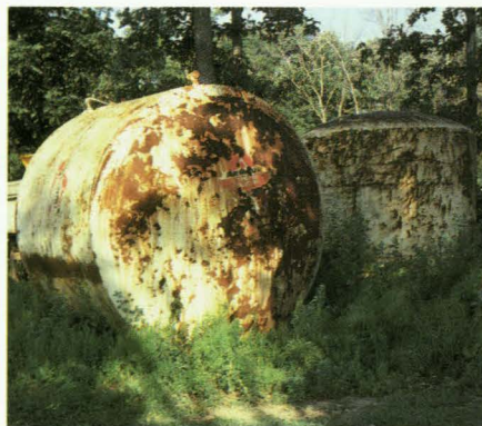
Underground storage tanks that are not properly installed may need to be dug up and replaced after only a few years.
