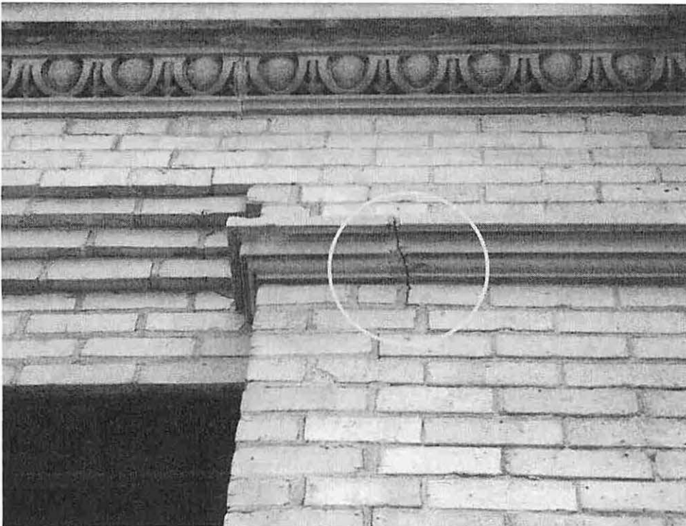
Figure 32: Cracked stone unit.
