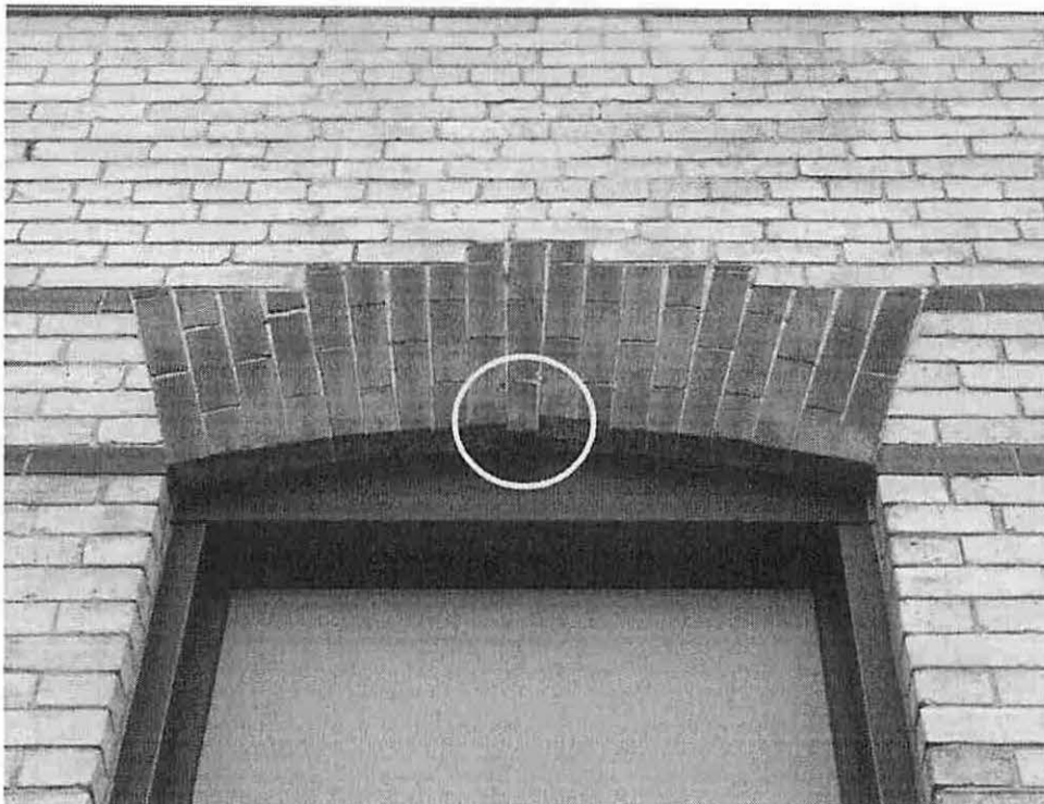
Figure 26: Loose brick unit.
