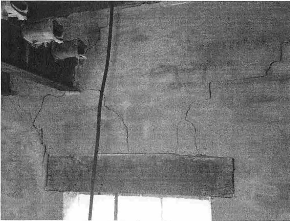
Figure 31: Interior cracking at lintel.
