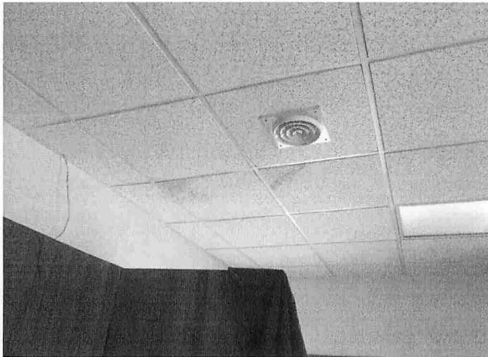
Figure 47: Stained ceiling tiles.
