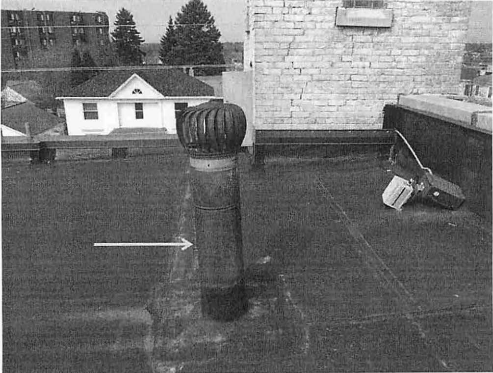
Figure 12: Corroded metal vent.
