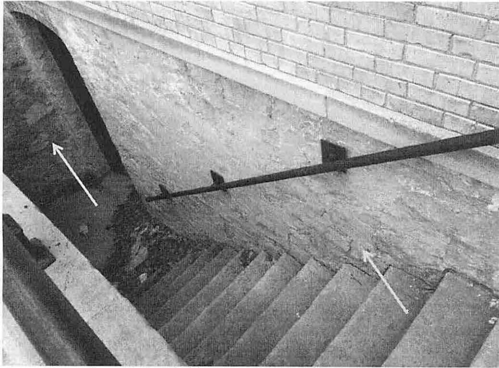
Figure 7: Deteriorated foundation walls.
