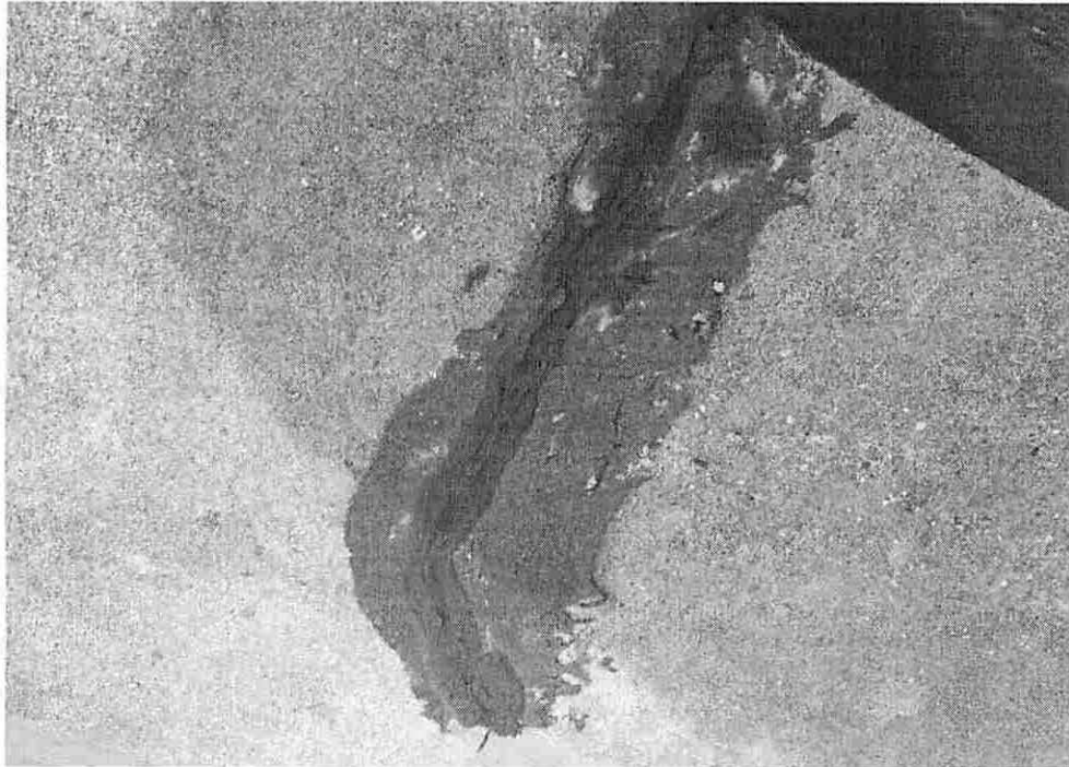
Figure 9: Deteriorated stone coping sealant.
