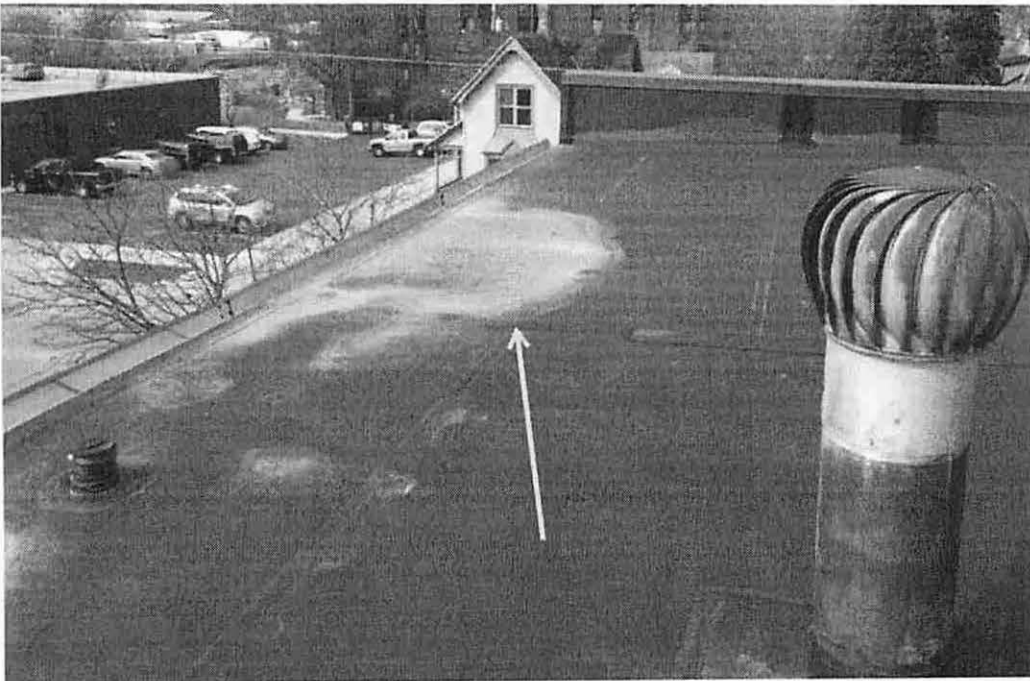
Figure 18: Ponding at south roof edge.
