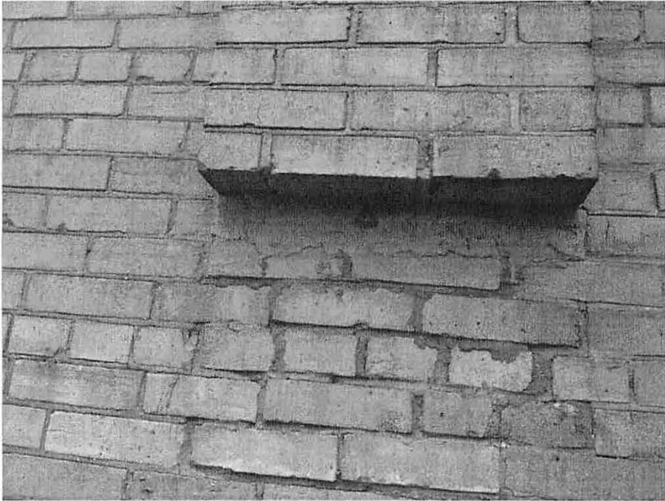
Figure 27: Deteriorated mortar joints.
