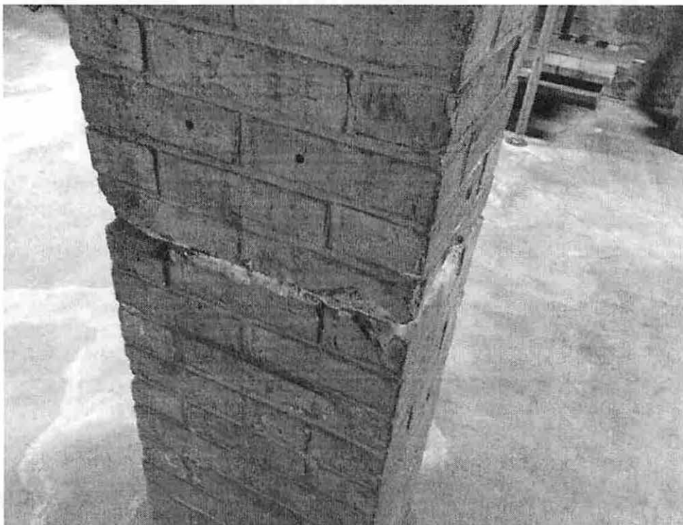
Figure 42: Brick deterioration; Deteriorated mortar joints.
