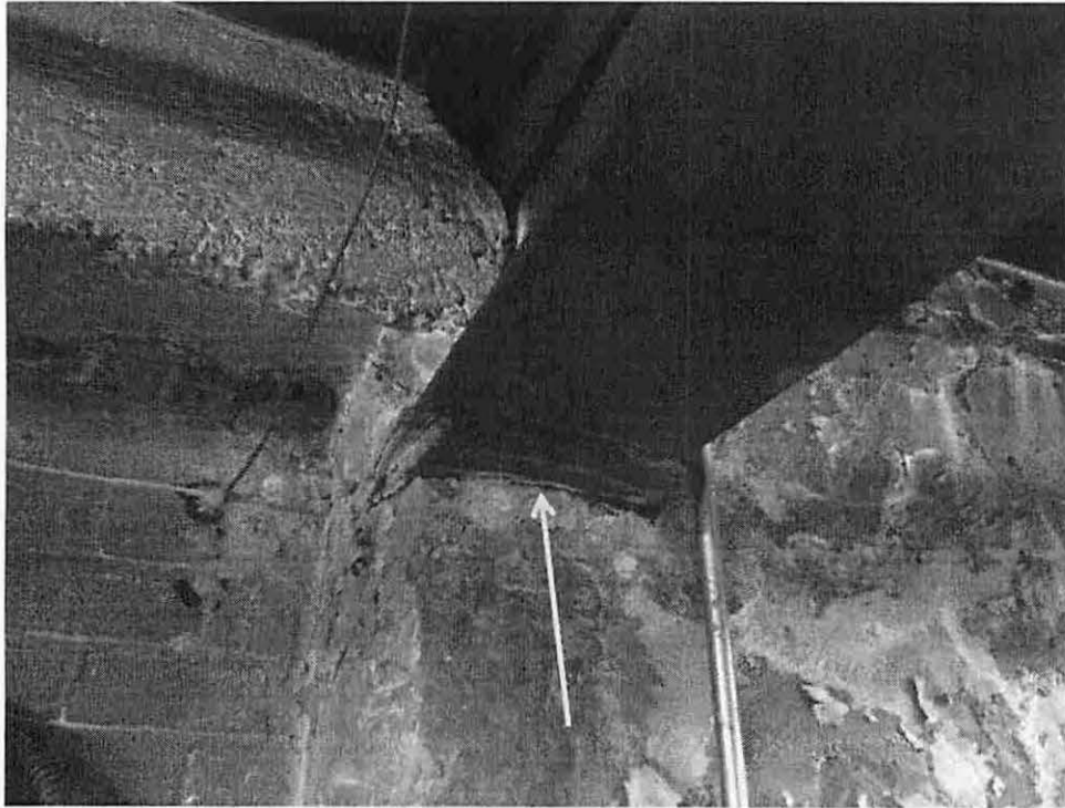
Figure 37: Corrosion of steel beam.
