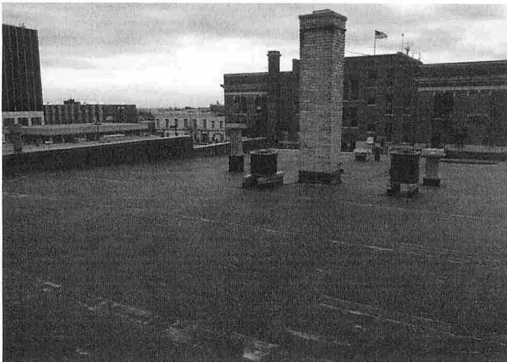
Figure 8: Full adhered EPDM roof system.
