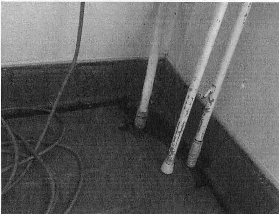
Figure 50: Unsealed penetrations allowing leaking into basement.
