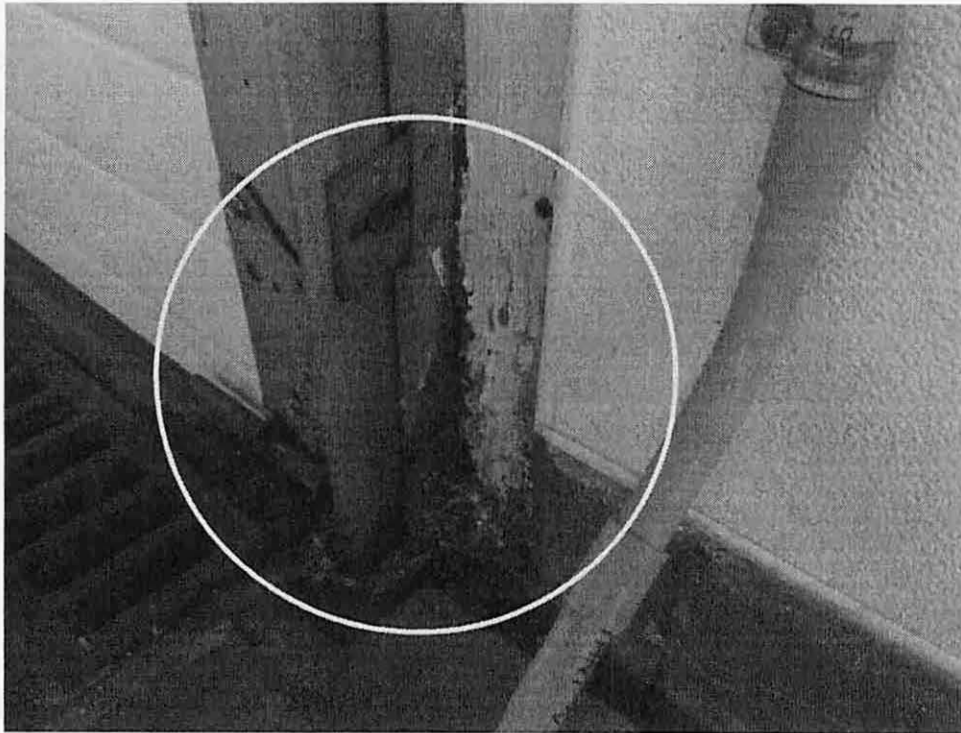
Figure 49: Deterioration of wood trim at garage door.
