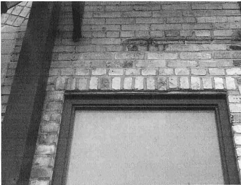
Figure 30: Corroded steel lintel.
