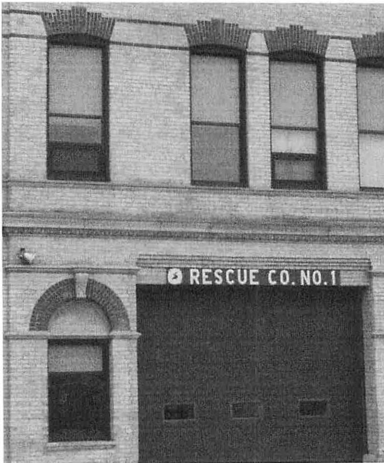
Figure 20: Typical window systems.
