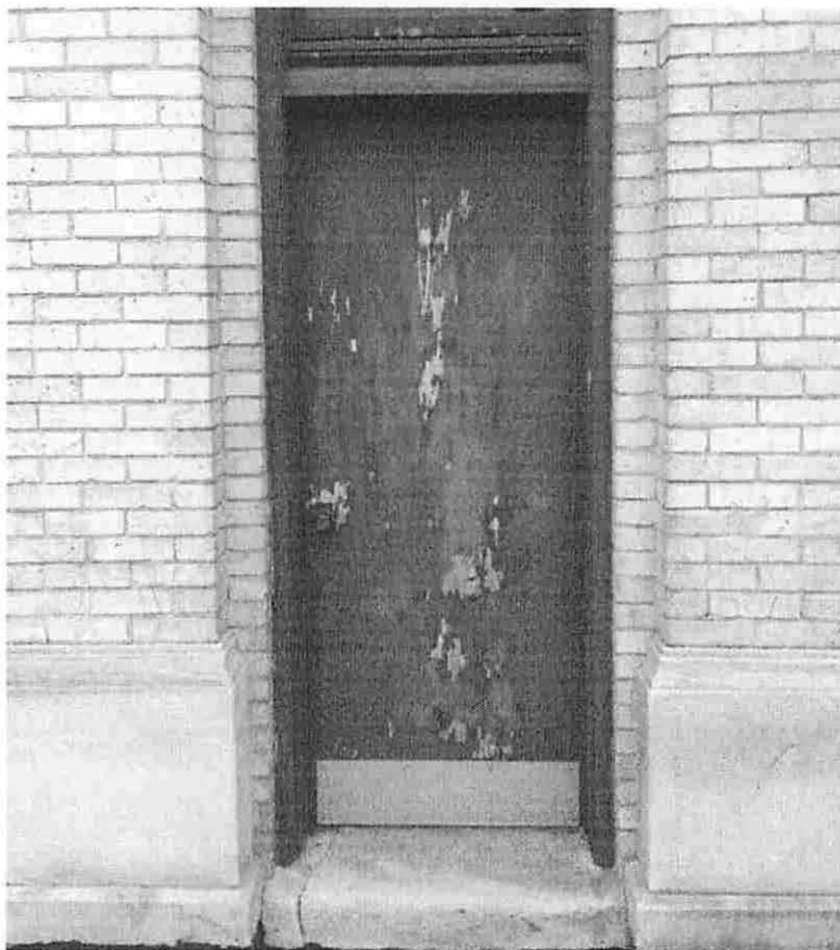
Figure 23: Deteriorating wood door.
