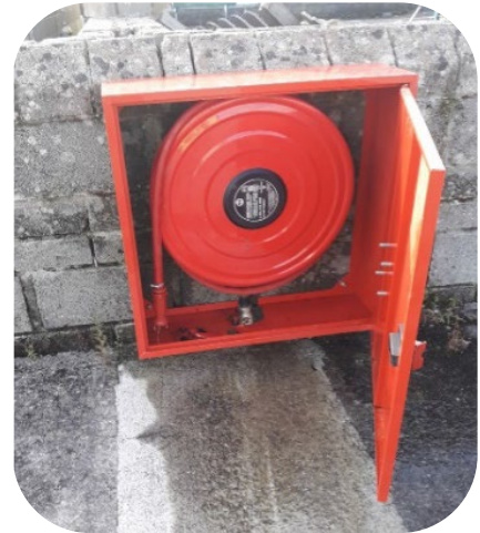
Fire Hose Reels Installed at Tuam Halting Site
