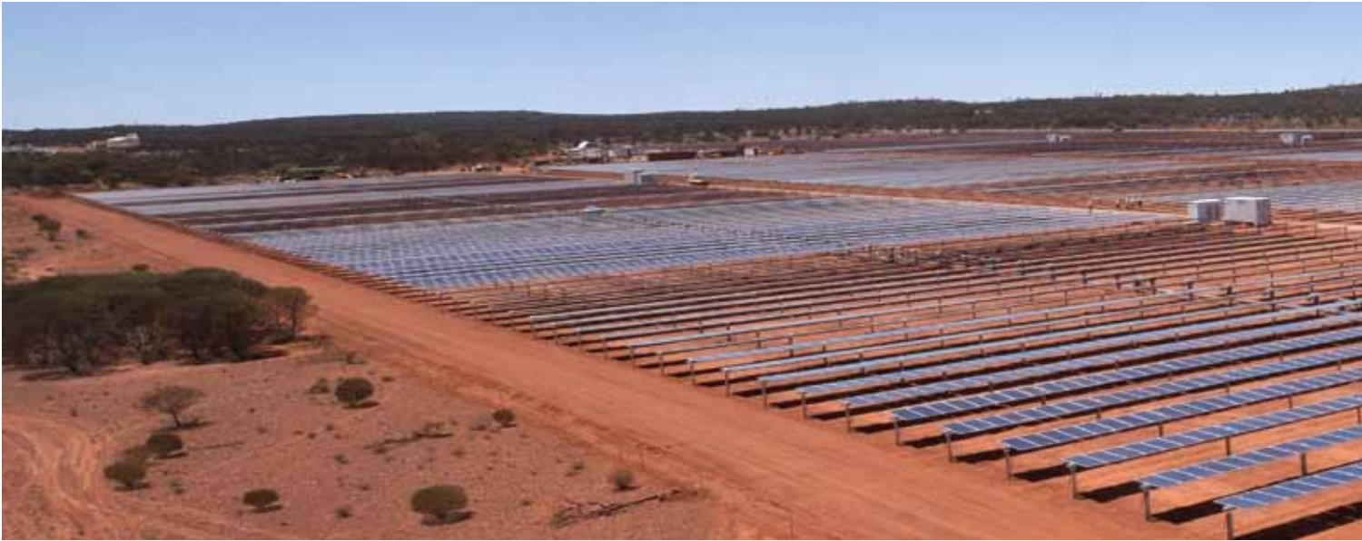
The remote location added to the labor and logistics required on the installation, a factor other EPCs may underestimate, says juwi Australia.
