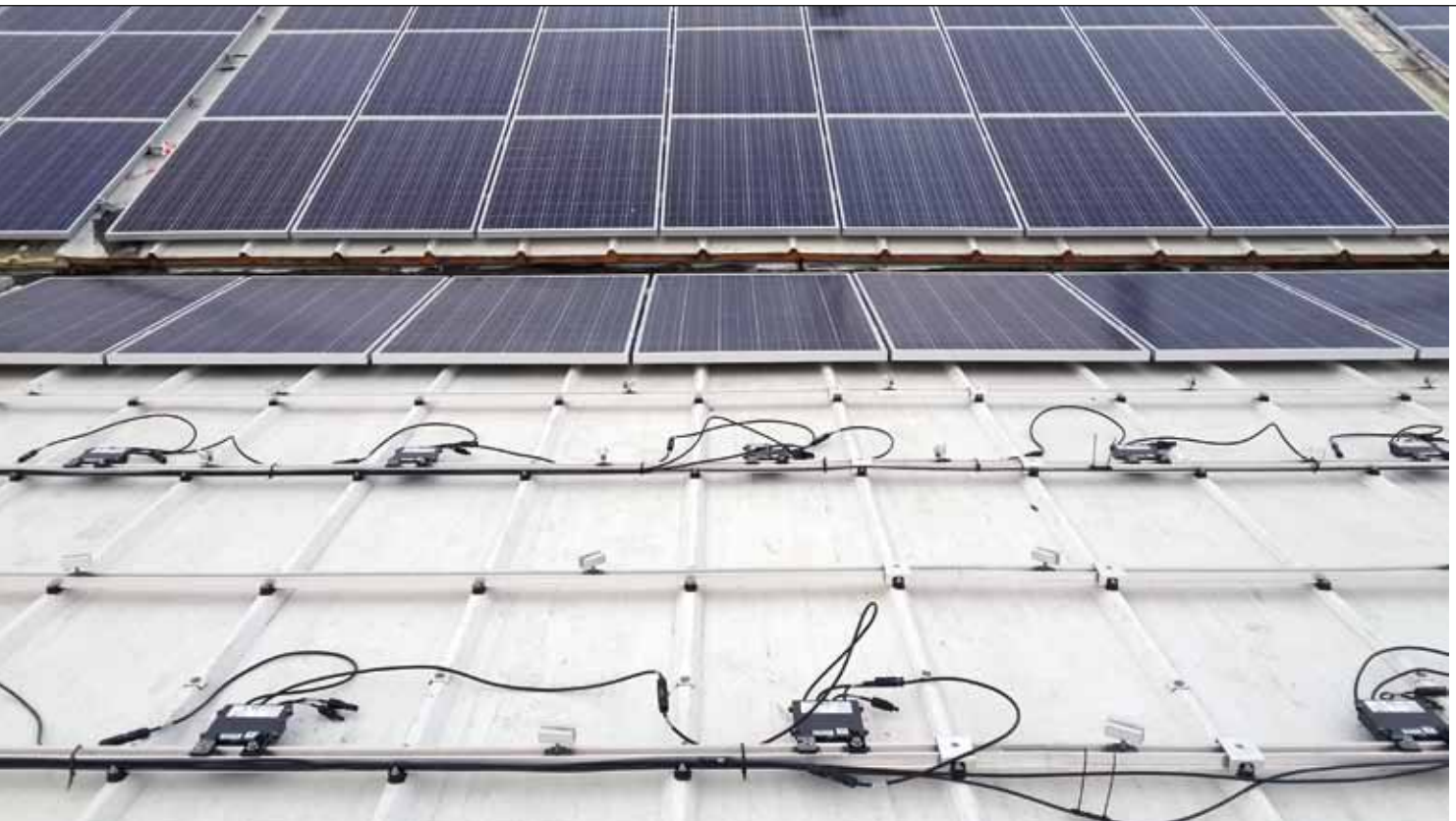
Module level power electronics are an increasingly common sight on solar rooftop arrays, with DC optimization technology nudging ahead of microinverters thanks, in part, to the flexibility these products offer.
