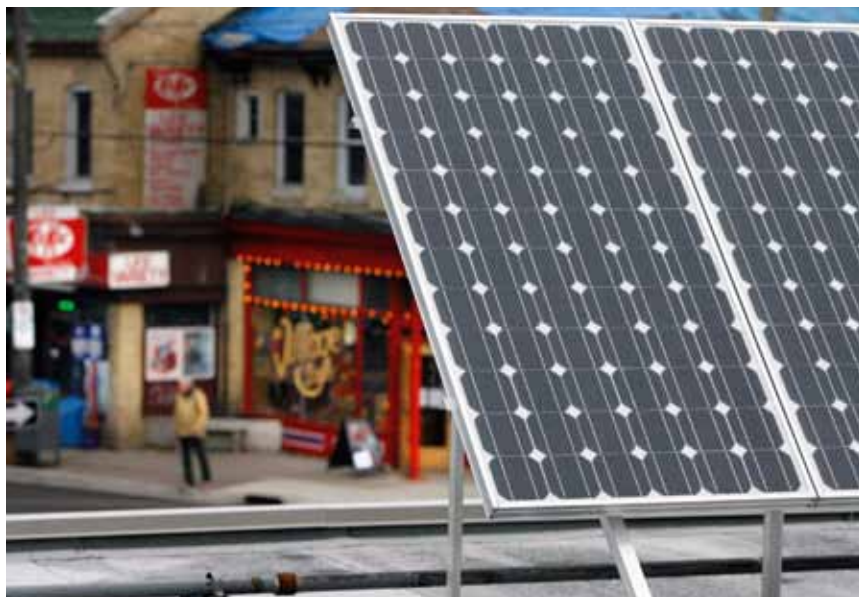
Rooftop solar PV is an increasingly common sight across the U.K., with the residential sector proving particularly fertile as customers were attracted by generous FITs prior to recent subsidy cuts.
