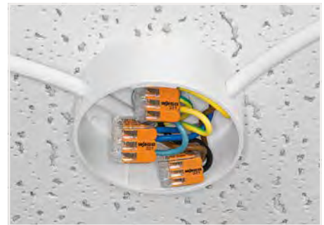
Lighting distribution in a ceiling canopy
