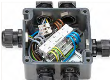
Wiring example in an Ex e junction box Labeling is performed via marking strips (210-334) and pen or continuous labels (210-834), which is printed via Smart Printer (258-5000).
