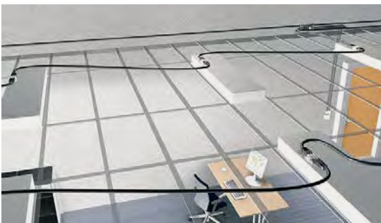
In suspended ceilings
