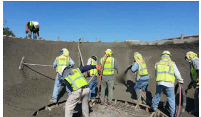
Fig. 3: Over-vertical pocket skate feature. 2018 Outstanding Shotcrete Award in the Pool & Recreational Project category
