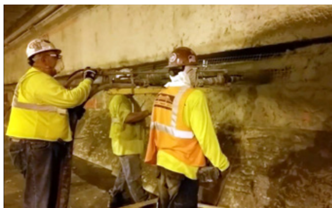
Nozzleman innovation for fireline encapsulation, 5-feet off the ground, at the Queens Midtown Tunnel. (2019 Outstanding Shotcrete Award)
