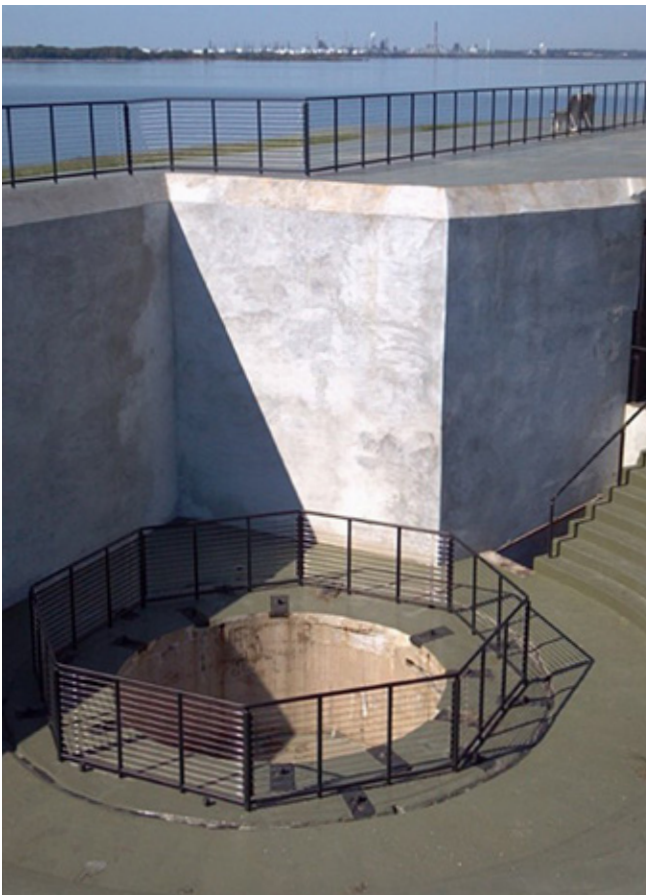
Historic rehabilitation of the battery walls and stairs at Fort Mott State Park, utilizing a mix design to match the existing composition and texture. (2012 Outstanding Shotcrete Award, Honorable Mention)
