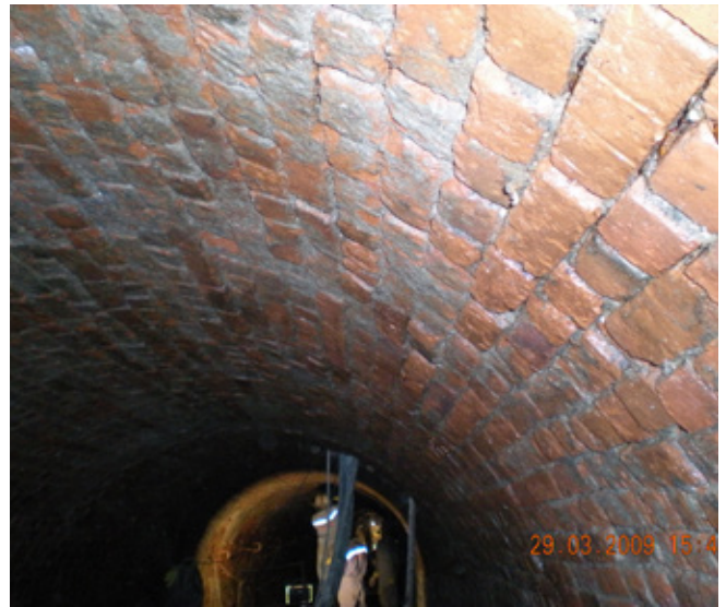
Fig. 3: Erosion of mortar joints
