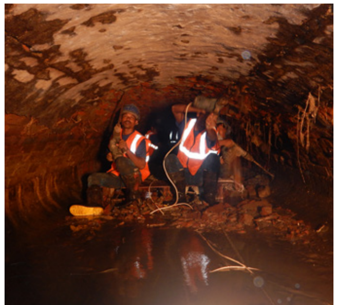
Fig. 4: Root penetration through masonry lining
