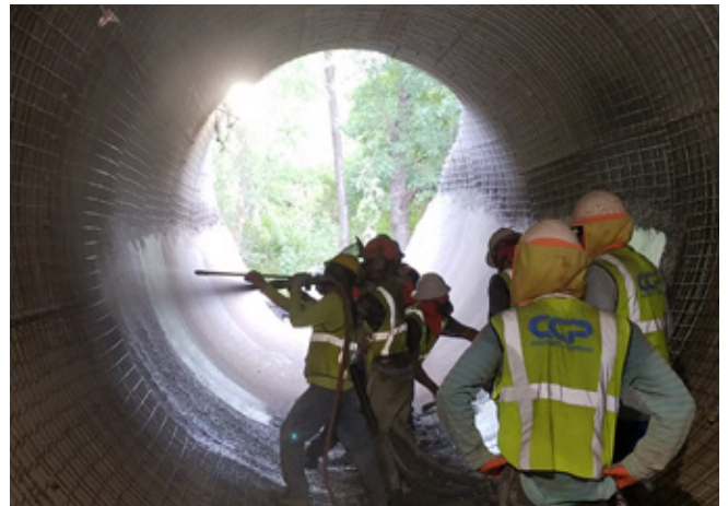
Fig. 3: TXDoT project calling for a 4 in. (100 mm) shotcrete lining of over a 172 ft (52 m) long, 14 ft (4.3 m) diameter corrugated metal pipe (CMP).
