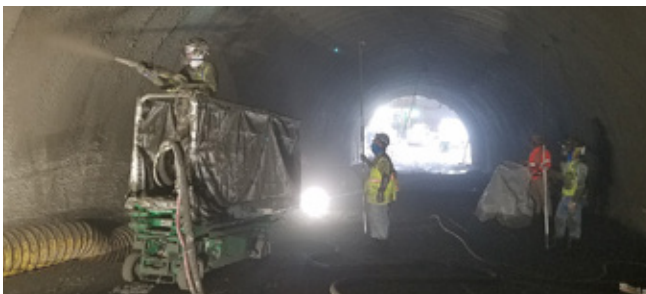
Fig. 2: Initial and primary shotcrete tunnel linings for the Houston Museum of Fine Arts. The 200 ft (61 m) tunnel in will soon be the newest art exhibit space.
