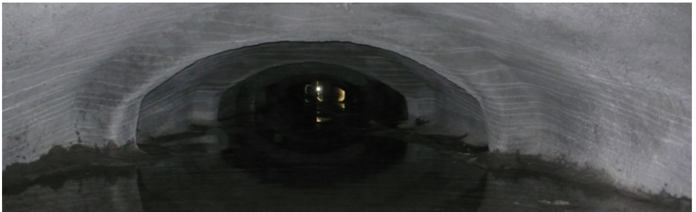
Fig. 1: Completed repair of the storm water drains in the City of Mumbai, India, that are over a century old and were constructed of brick arch masonry during the British Era
