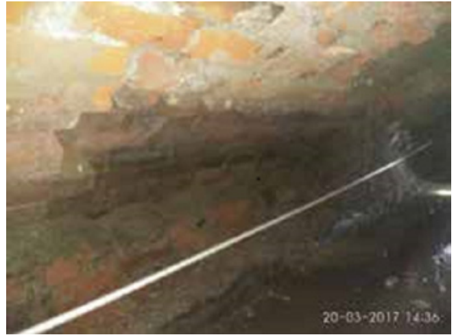
Fig. 2: Delamination and spalling of brick lining
