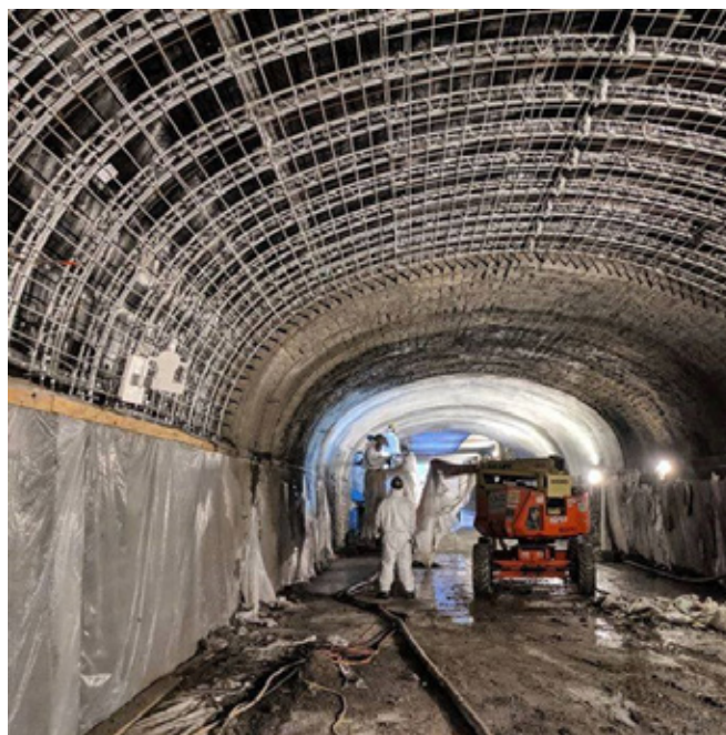
Lattice girders over waterproofing membrane, to support 9 to 12 inches of overhead shotcrete for the reconstructed ceiling arch of the Park Avenue Tunnel.
