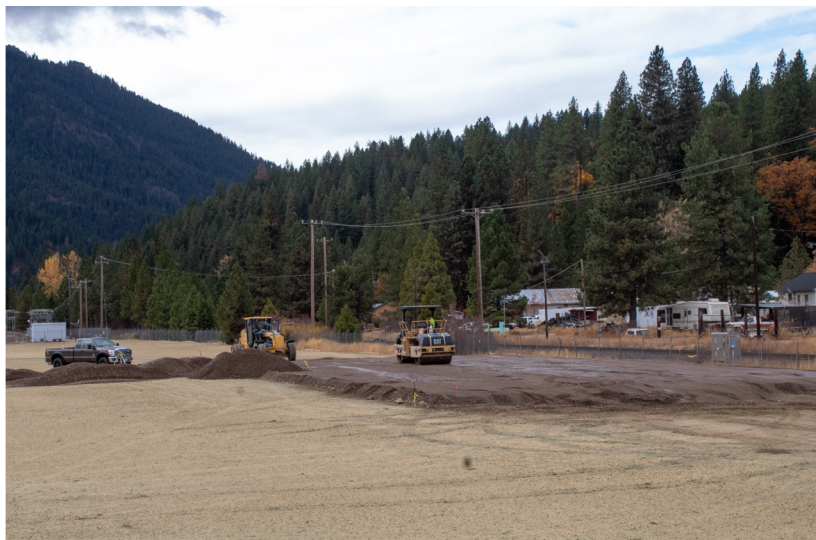
Brownfield remediation work to create a wood chips storage shed at Indian Valley Wood Products Campus in Crescent Mills, California
