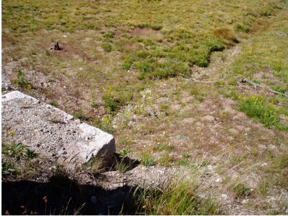
Figure 2-19. Example of downcutting observed in meadow directly downstream of culvert.
