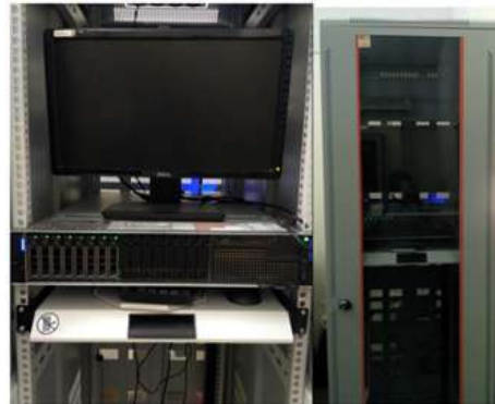
Fig 6.4 Deep Learning Servers Dell EMC R740 and R 750
