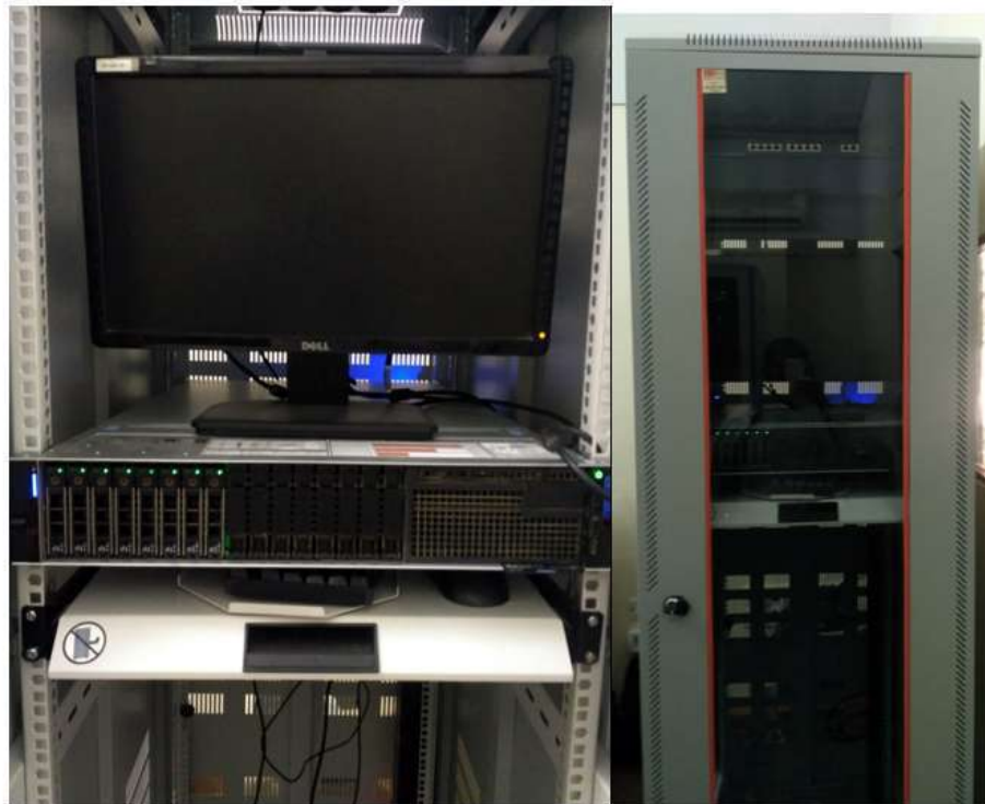
Fig 5.26 Deep Learning Servers Dell EMC R740 and R 750
