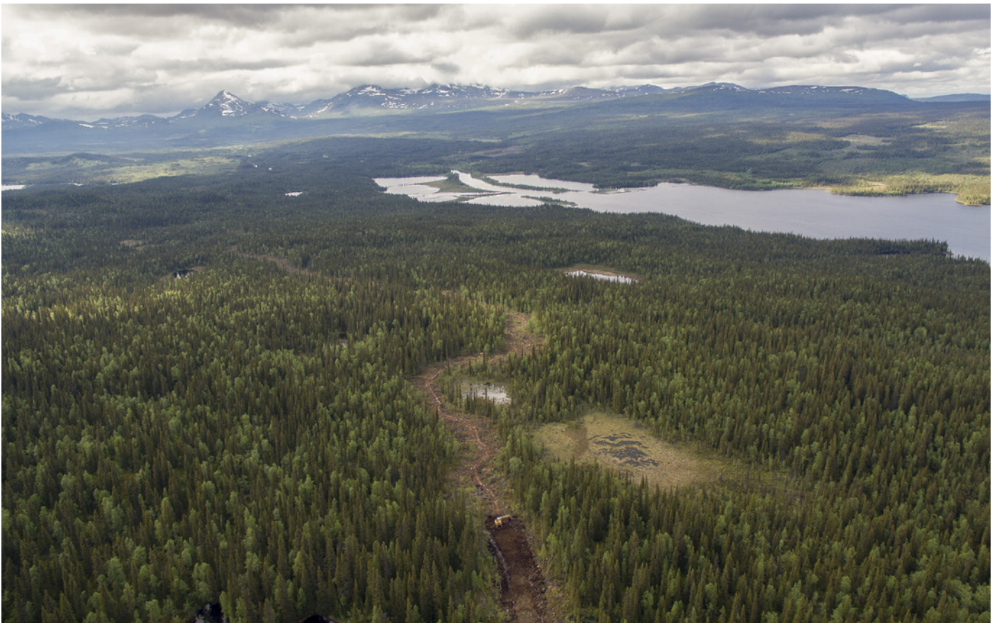
Figure 7. Ongoing road construction through old-growth forest, mires and creeks. The caterpillar excavator can be seen digging in the lower middle section of the photo.
