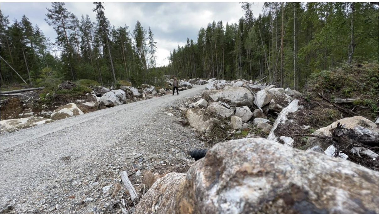
A forest vehicle road has been built right into a untouched natural forest area of 200 hectares at Vargtjärnen, Ånge municipality. (WGS84: 62.57162, 16.06995). Photo: Private.
