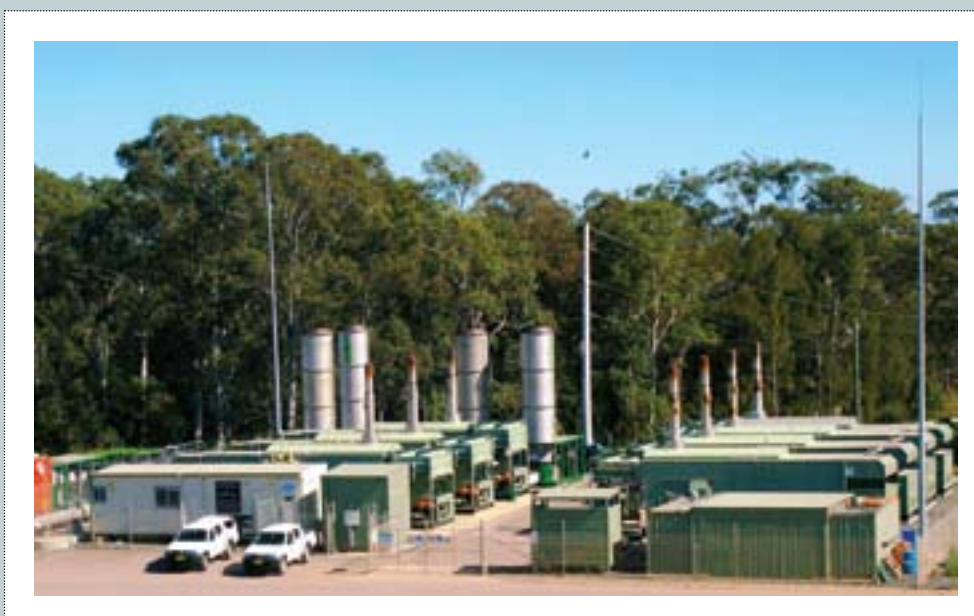
LMS Generation's jointly owned landfill gas renewable energy facility at Eastern Creek, NSW – Australia's largest built this decade.
