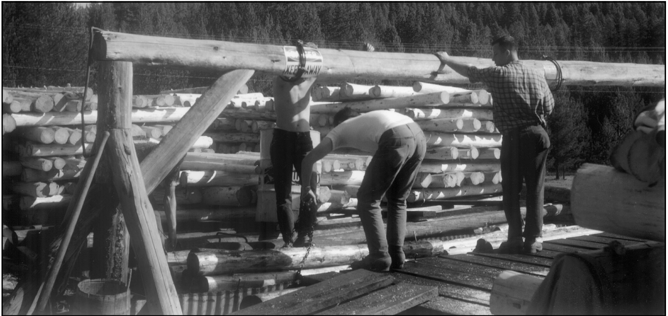
Thorn Creek Detail soaking fence posts in tank of preservative. (Courtesy Denis Symes)
