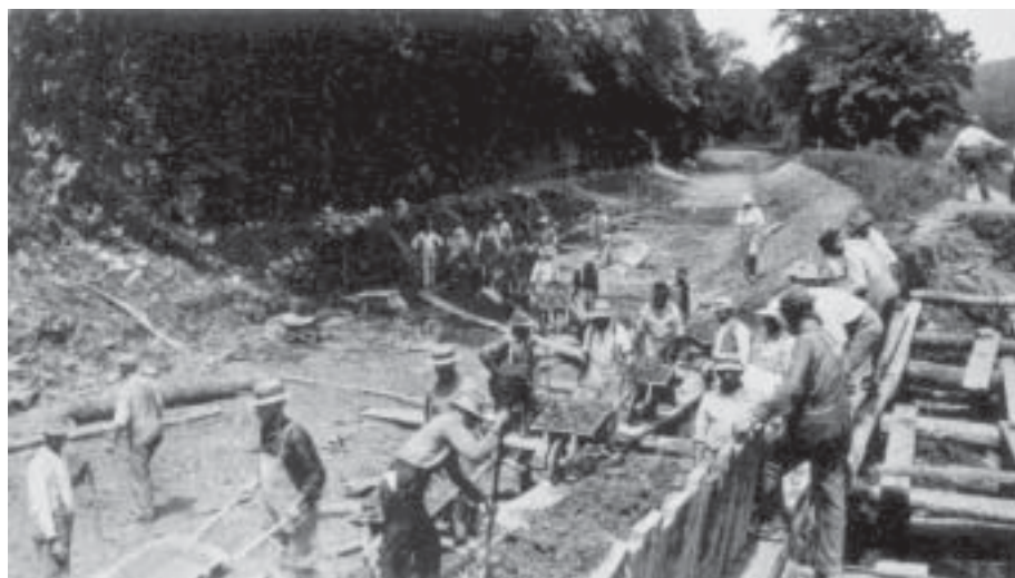
Flood damage in 1903 near Lumberville. Photo from Canal History and Technology, Easton, PA.
