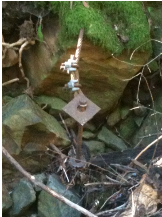
Figure 8: A disconnected bolt from CDFW LWM.
