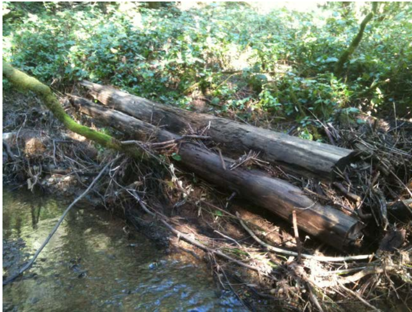
Figure 9: Two attached pieces of CDFW LWM that has broken apart from original anchoring. These pieces are loose and will likely move in periods of high flow.
