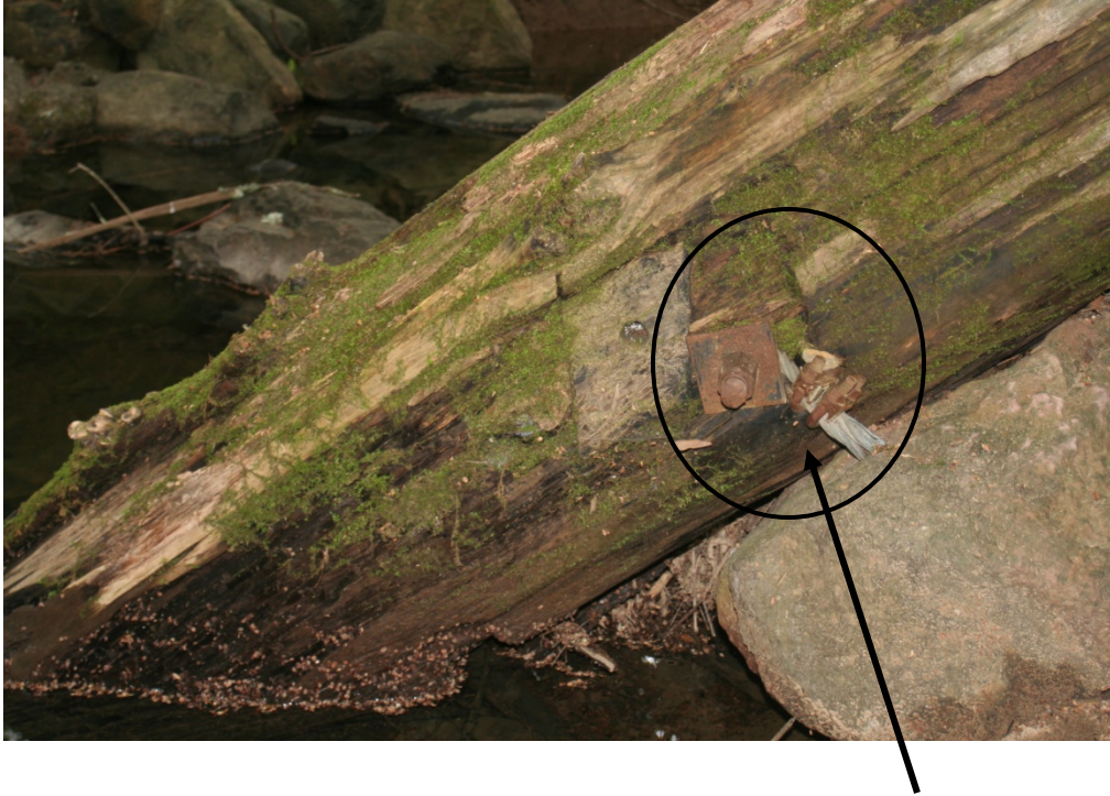
Figure 7: Felta Creek (F1b): an example of LWM attachment to boulder using bolts and cable
