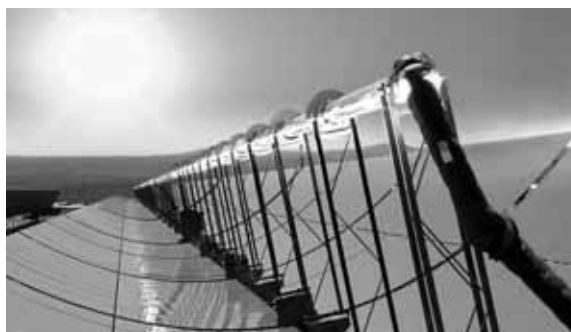
Photo courtesy of SCHOTT. Receiver for solar thermal power plants. Successful test run: The receiver from SCHOTT has already proven itself as a part of a string of collectors at a parabolic trough power plant in California.
