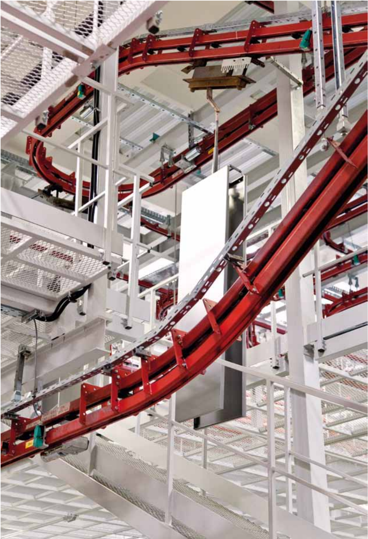
Hanging conveyor system for transport of semi-products from powder coating to assembly and the insulation department
