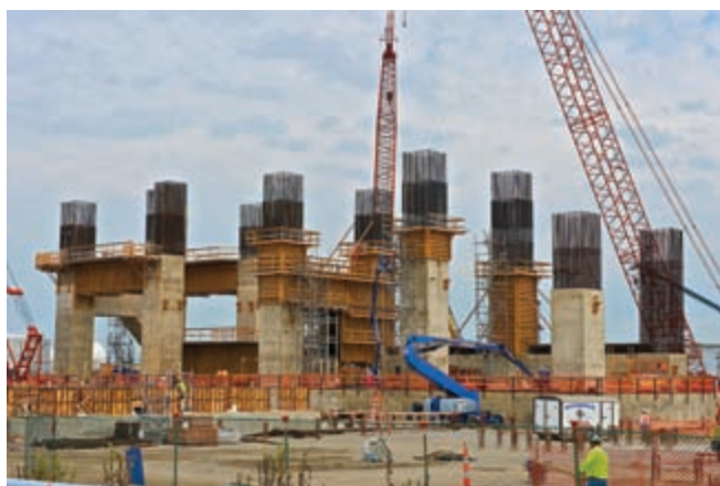
Left: Concrete pylons are poured to support the coke drums and derrick structures.
