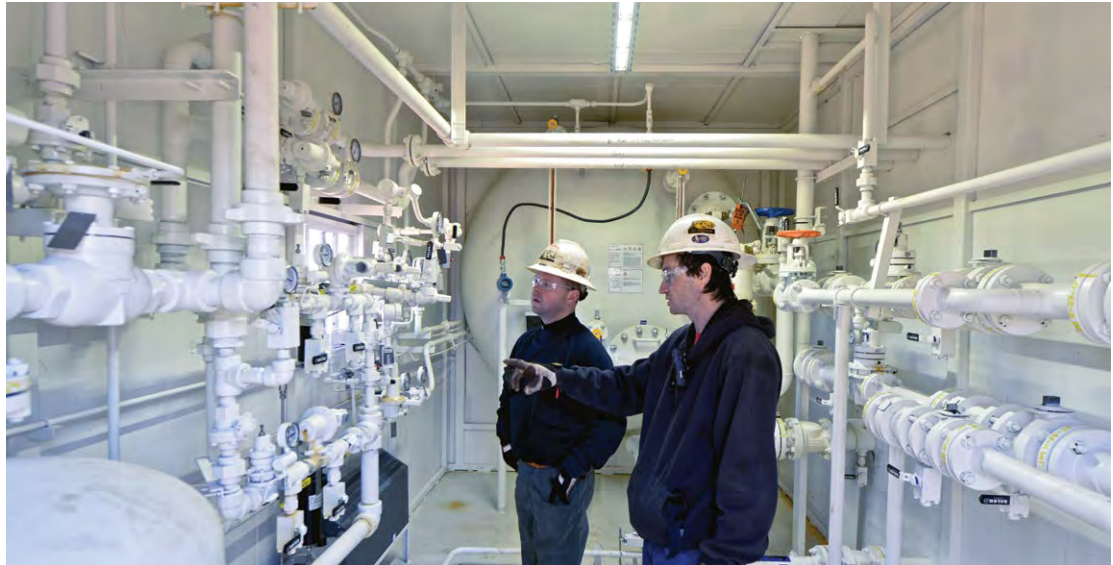
Jon Lowry (left) and West Neville examine piping in a bulk separation plant.
