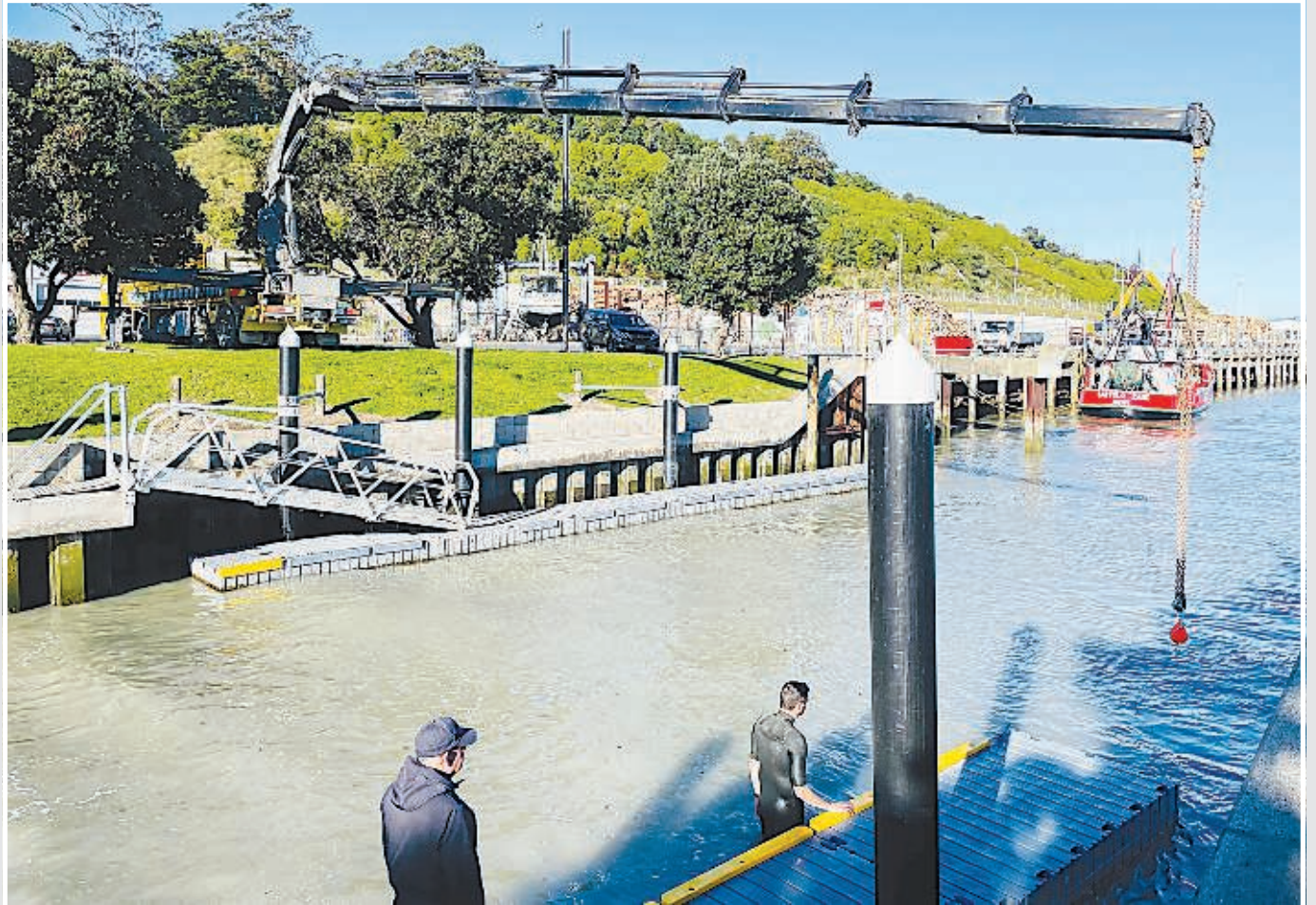
PONTOON PROBLEMS: A crane removes two sections of the broken pontoon out of the water at the Inner Harbour this morning ahead of a heavy swell forecast for tomorrow. Gisborne Hiabs was supported by a diver in the water and harbourmaster Peter Buell at the Inner Harbour boat ramp. Gisborne District Council liveable communities director Michele Frey said the contractor who developed the pontoon would be in Gisborne in two weeks. "This will enable us to assess the issue and to make repairs with a view to secure the pontoon for future use." The $400,000 pontoon was breaking apart after heavy tidal surges over the weekend. Picture supplied
