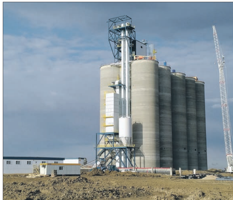
GrainsConnect is building four elevators in western Canada, including this one at Maymont, Sask. It is scheduled to open this fall. | GRAINSCONNECT PHOTO
