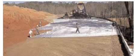
To complete this reinforced slope, 44,723m 2 (53,500yd 2 ) of the HS400PP and 43,495m 2 (56,000yd 2 ) of the HS800PP were installed as primary reinforcement.
