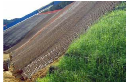
Placing geocell facing with topsoil infill for one of the shallow reinforced slopes
