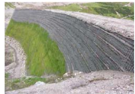
Wire mesh facing on the reinforced slope face with vegetation applied to the lower part of the slope
