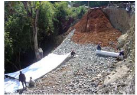
Placement of stone drainage blanket with Polyfelt® TS geotextile filter on top
