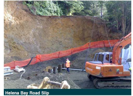
Helena Bay Road Slip
