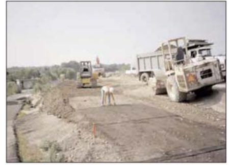
Miragrid* BXT, used as the primary reinforcement, is installed in 0.9 m (3.0 ft) embedment lengths.
