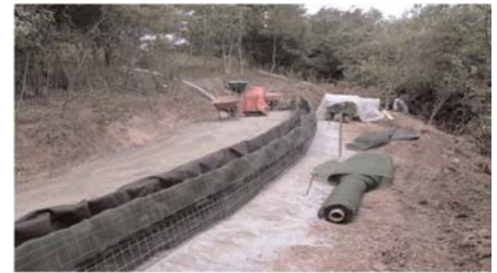
A welded wire wall is constructed with Miragrid® 3XT, Miragrid® 150N, and Miramesh® GR.
