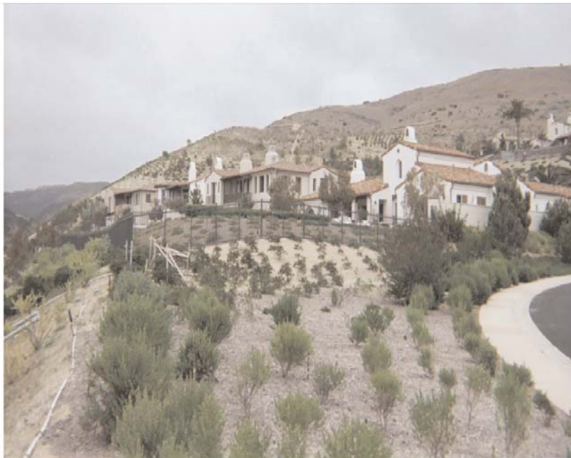
These premium lots were considered unbuildable. Miragrid® geogrids made it possible to develop this valuable property.
