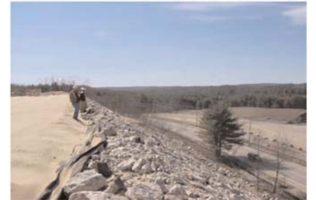
BELOW: The Miragrid® reinforced slope saved approximately 30% compared to the original SRW design.
