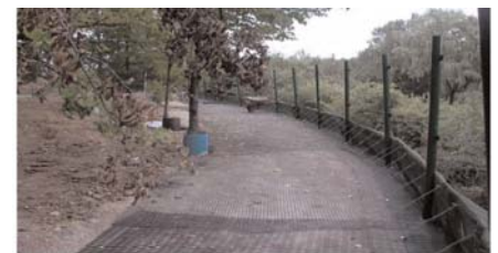
Each basket overlapped 100mm (4in.) Miragrid® 3XT was placed to the front face, then Miramesh® GR was installed along the wire struts.
