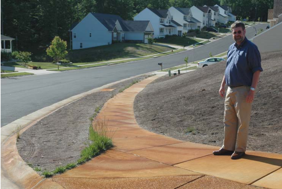
Lee Daniels, soil scientist and reclamation expert from Virginia Tech is shown standing on discolored side walk around house at the corner of Great Oaks Lane and Hickory Court. Grass is growing along the edge of the concrete probably because of the liming effect of the concrete.
