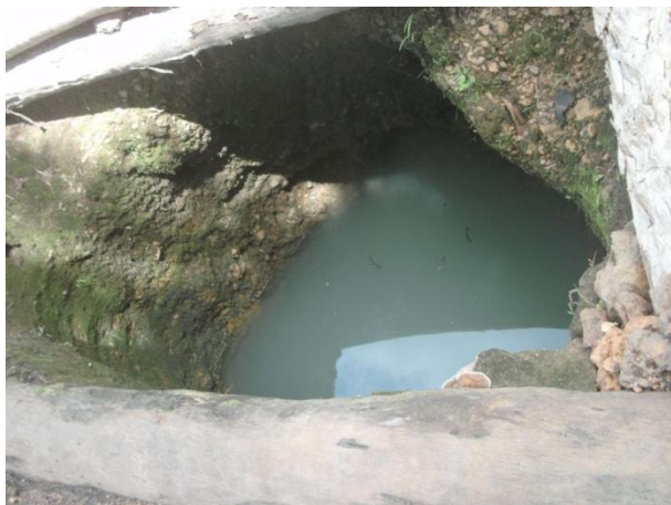
Figure 7 - An unprotected well in Kasserri
