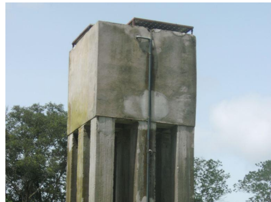
Figure 23 - Water tank in Gbendembu
