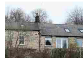
Water tabling on conversion
