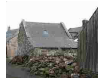
Water tabling on outbuilding
