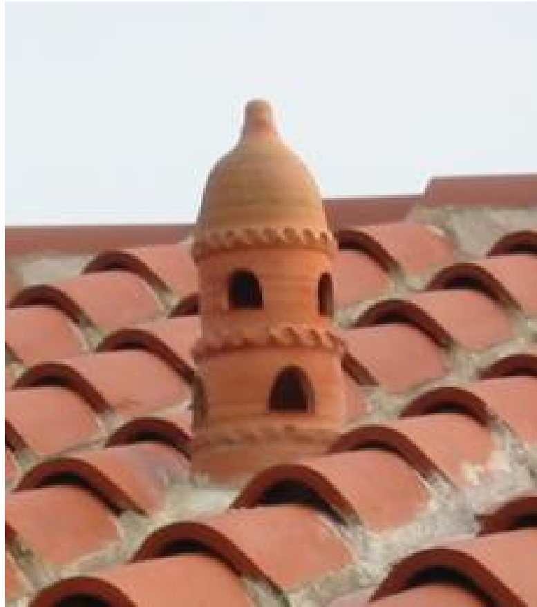
Plate 3: A chimney on a reconstructed Roman roof at South Shields, South Tyneside
