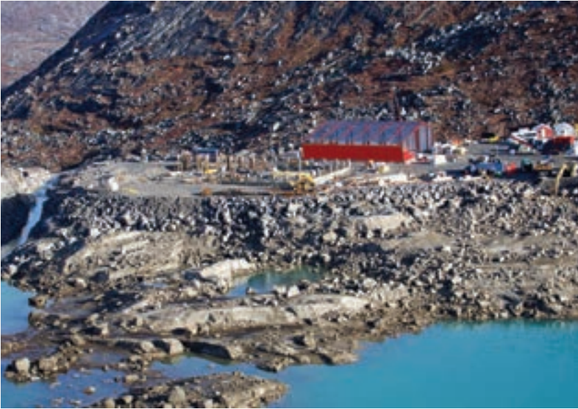
Figure 4: This aerial photo shows the construction of the processing plant and main workshop at the Aappaluttoq deposit, well underway. The processing plant will employ dense media and magnetic separation, as well as advanced optical sorting technology to extract the corundum. Since this image was taken in October 2015, the plant building has been completed. Photo courtesy of True North Gems Inc.
