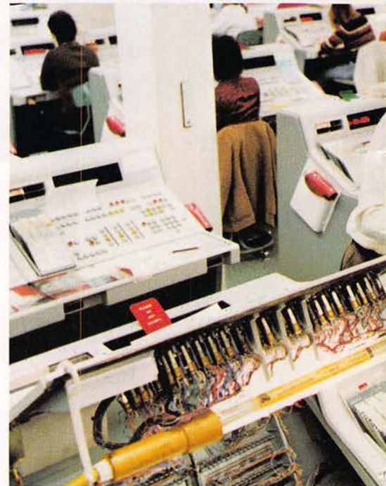
Top — Tony Severini explains crossbar wiring procedure to newcomer Barbara Murphy. Below — Joe Roche checks modification of N.J. Bell operator's position with installer Bill Tharp.
