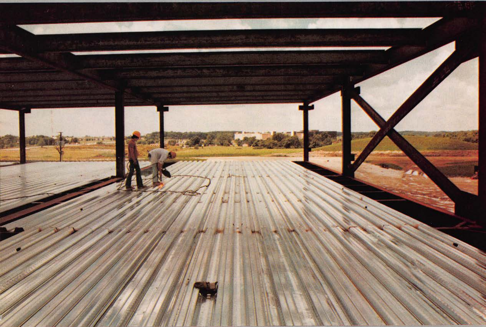
Following official groundbreaking ceremonies in 1979, workmen began positioning steel framework (left and above) in April at the site of the company's new Software Center in Lisle, Ill.
