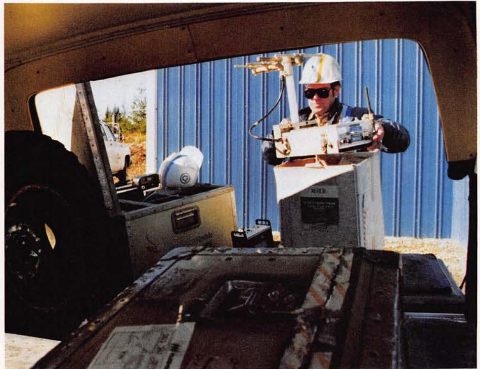
Above—Bob Herring from the Denver Turnkey group unloads radio gear at West Harness. Left—he directs the antenna crew working on the tower.
