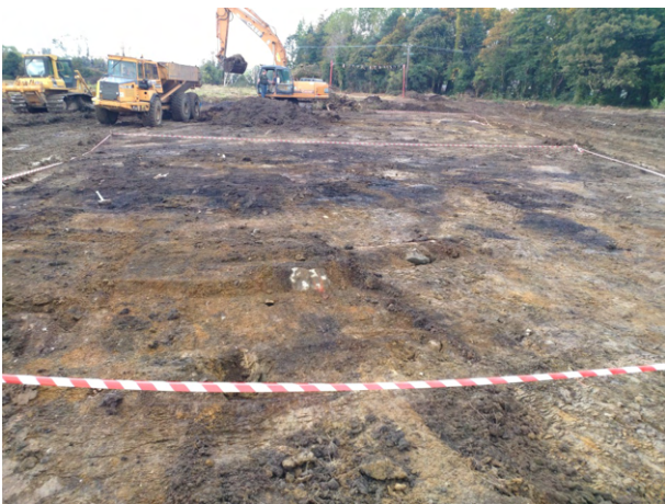
View of the north end of Area 1 after stripping, looking north (top)
