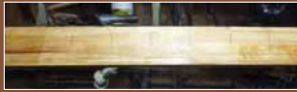
2 - First stage of the marking out showing both ends and the start of the grid layout
