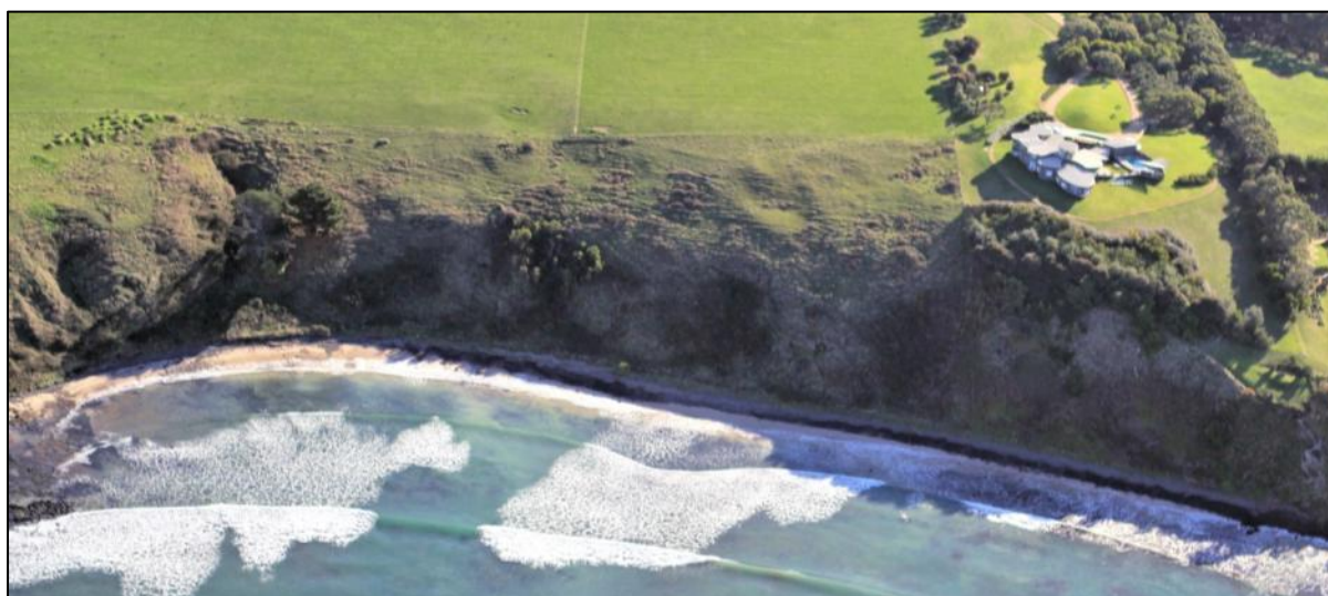
Figure 3-45 Platform Beach and Bluff Susceptible to Reactivation due to Sea Level Rise, Flinders/Shoreham (Photo N. Rosengren 8 June 2013).
