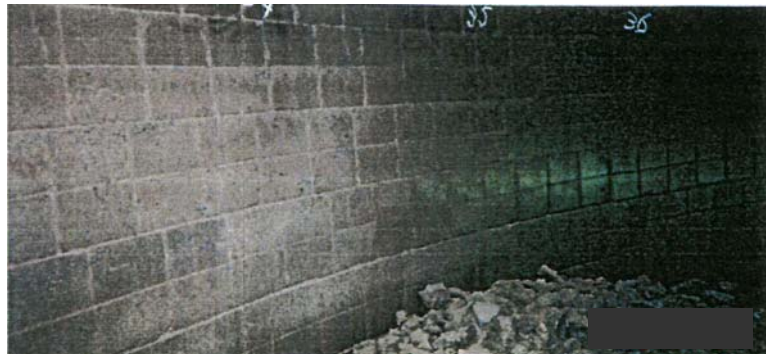
Figure-9.2 Photograph of cooling chamber refractory after 8 years operation (After change of the refractory quality)
