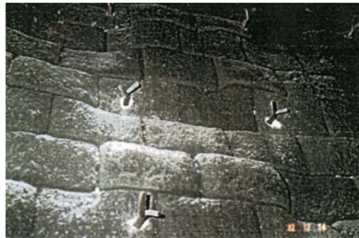
Figure-9.1 Photograph of cooling chamber refractory after 1 year operation (Before change of the refractory quality)
