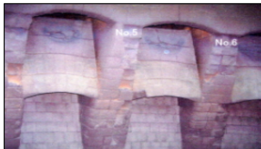
Figure 13: Photograph of refractory of Double flue after 5 years and 8 months operation (Using high durability refractory)
