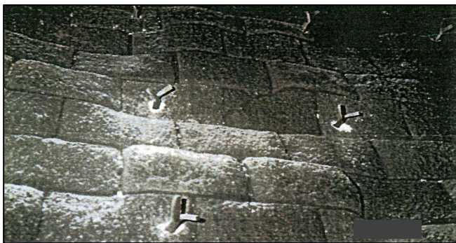
Figure 8.1: Photograph of cooling chamber refractory after 1 year operation (Using conventional refractory)
