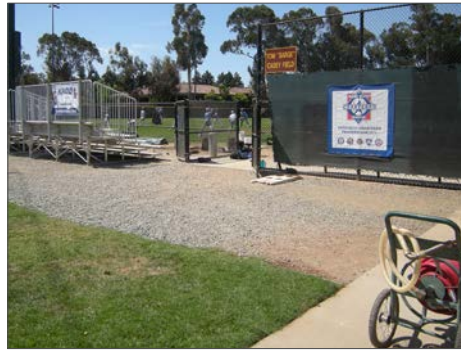
B | No ADA access to bleachers
