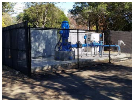
D | Utilities water well
